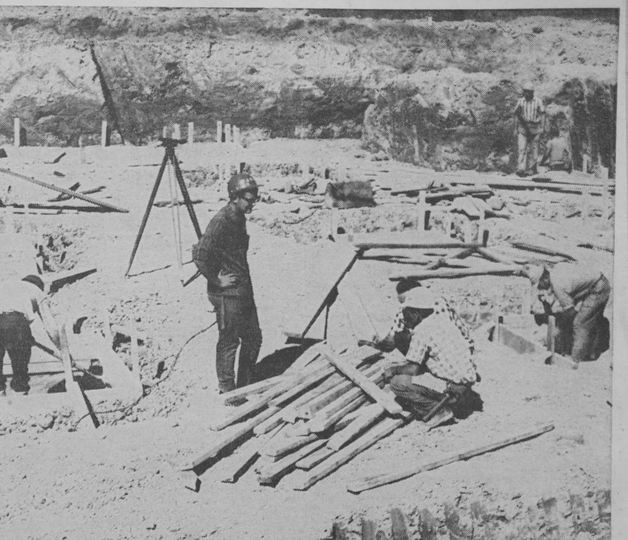
Full Speed Ahead Foundations are well underway at the York Central District Hospital on the Maple Sideroad. Seen above are some of the workmen putting the finishing touches to the cribbing under the kitchen at the rear of the structure. The hospital is expected to be completed late next year. (Staff photo)
