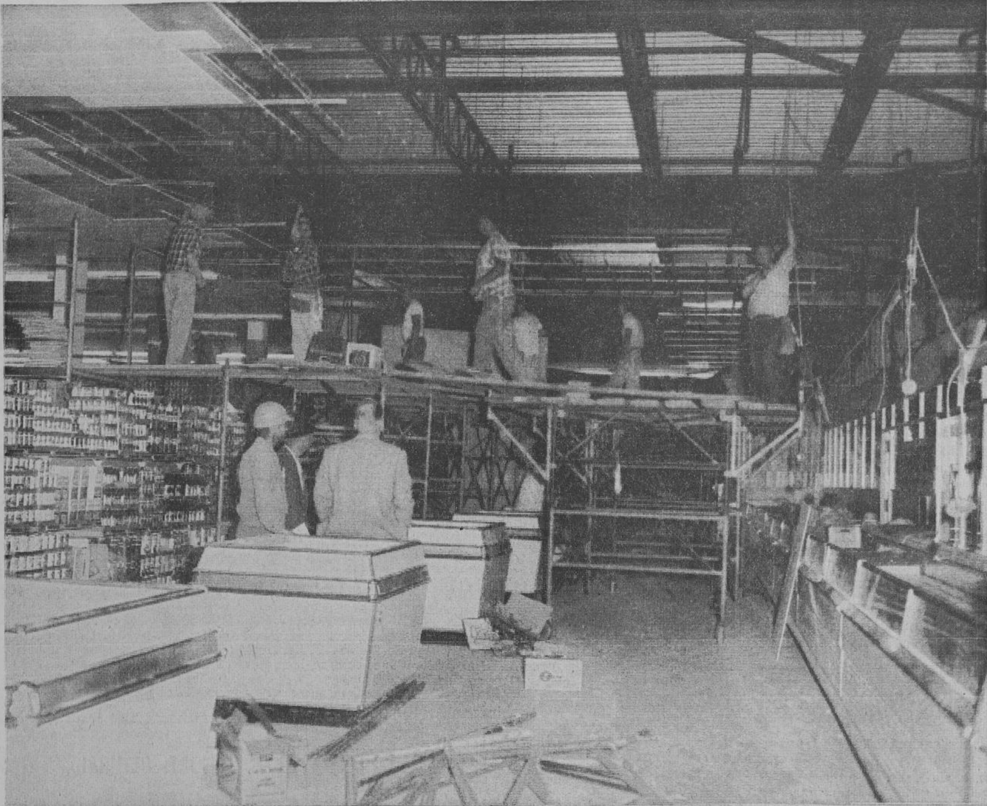
Workmen can be seen repairing the recent damage to the ceiling of the G.E.M. Department store located on Yonge St. in Highland Park. The acoustic tile and lighting in an area approximately 100 feet by 30 feet collapsed resulting in injuries to six people. The most seriously injured was
