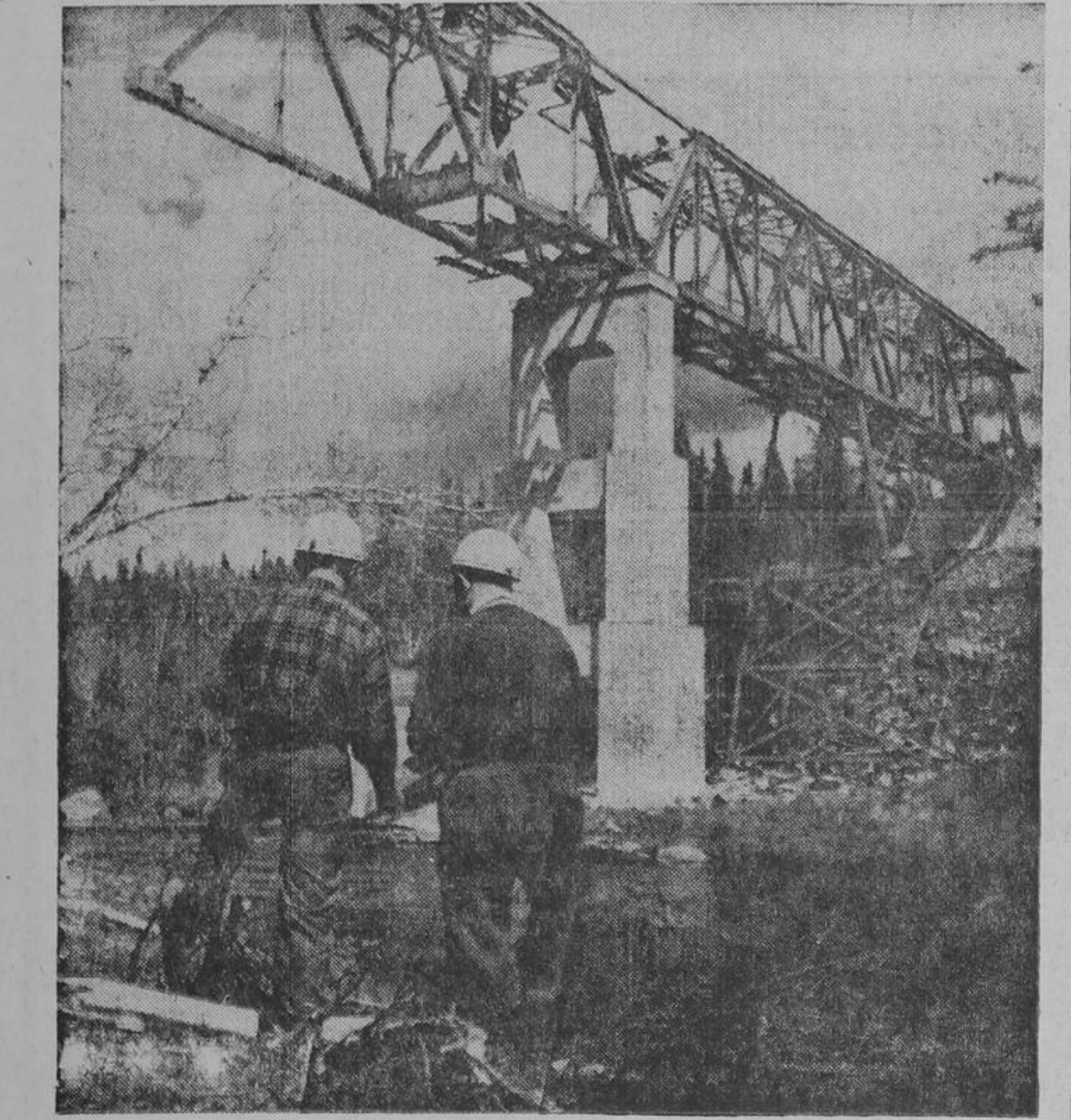
BRANCH LINE NEARS COMPLETION — One of the most difficult construction problems faced by Canadian National Railways' engineers in the building of a new 294-mile C.N.R. branch line to link mineral-rich Northern Quebec with the industrial areas of the province was the 400-foot bridge spanning the gorge of the Cran River. The bridge, 32 miles northwest of St. Felix, was constructed by the cantilever method. To transfer workers & materials to the opposite side of the deep gorge, a needlemast was erected to support a cableway similar to the breeches-buoy technique employed to transfer men between ships at sea. The first section of the line between Beattyville and Chibougamau was opened in 1957 and it is expected the second section from Chibougamau to St. Felix, of 133 miles will be opened late this year. The new town of Chibougamau is now a thriving municipality of 4,000.
