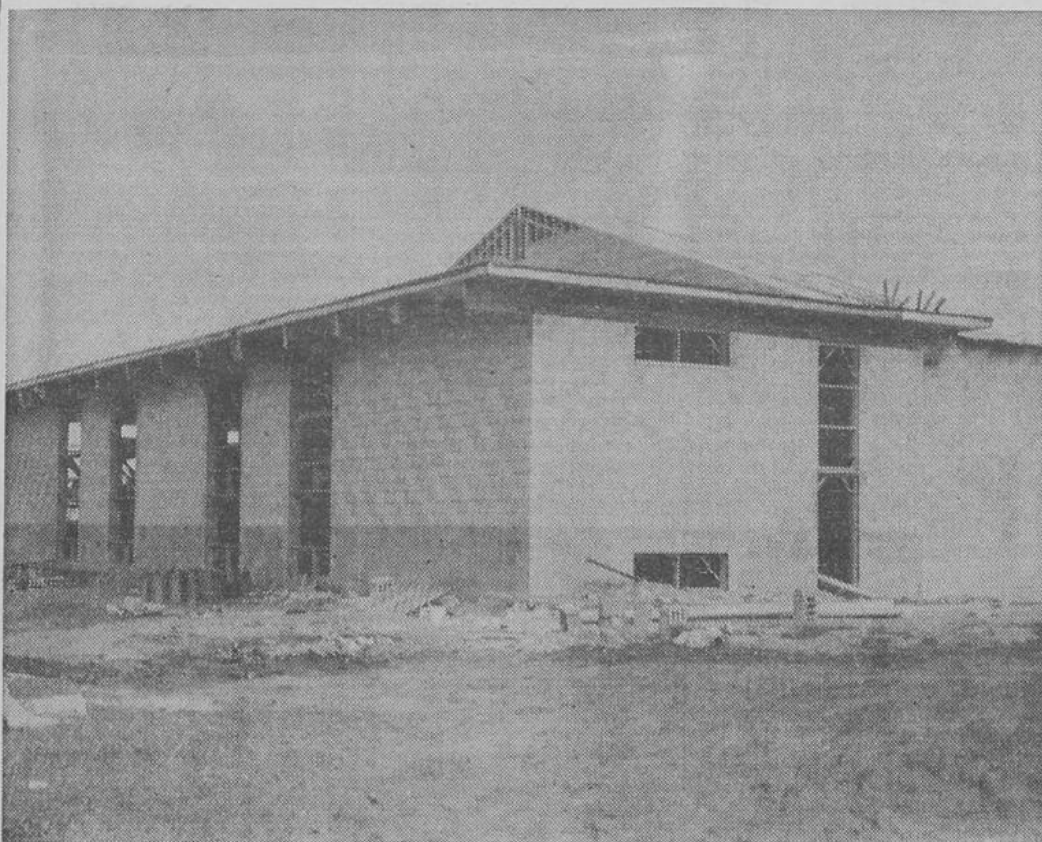
The above photo shows the progress in construction of the Richmond Hill Curling Club's fine new building. View of the rink structure shows the lounge, the photo taken from the north-west side.
