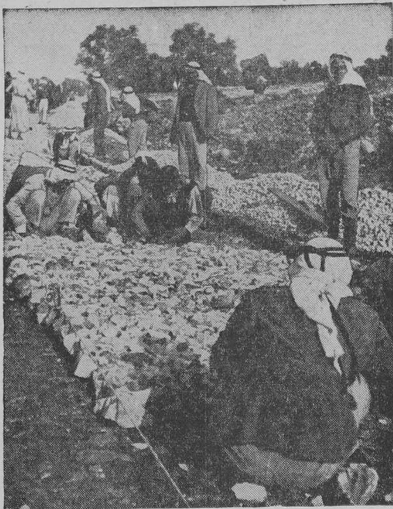
SINCE the partition of Palestine thousands of Arabs have taken refuge in neighboring countries. The U.N. Relief and Works Agency for Palestine tries to provide opportunities for a better future. Here is a group of them working on an UNWRA road building project.
