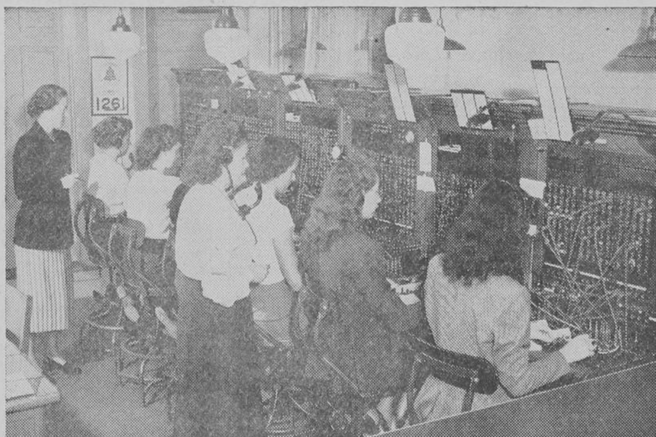
In contrast, the expanded switchboard at the local exchange today shows part of the operating staff of twenty who handle telephone traffic in Richmond Hill. At extreme rear left is Miss Alba Thompson who is the chief operator here. The six positions shown here represent 100 per cent increase in facilities within the last three years, and a seventh is to be added shortly.
