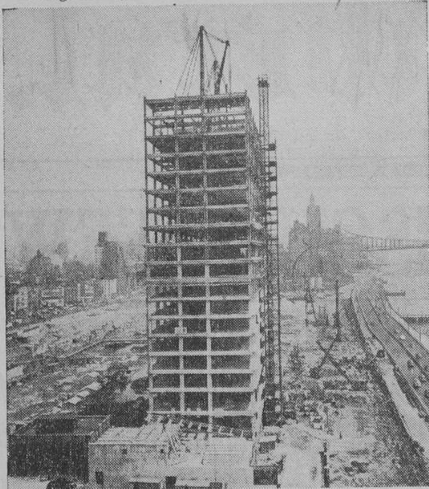
Steelwork on eighteen of the 39 stories of the United Nations Secretariat building in mid-Manhattan, New York, was completed in July when this picture was taken. A contract was signed by U.N. and the American Bridge Company for the furnishing and erection of structural steel for the meeting hall area of the Permanent Headquarters. The contract calls for 10,500 tons of structural steel at a cost of $2,225,000. Delivery is to be made by next October, and erection is expected to be completed by April or May 1950.
