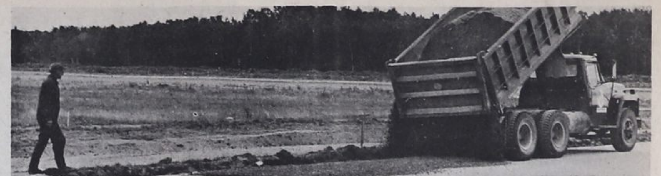
Work on the runway resurfacing project is nearing completion at the Huronia airport field in Tiny Township. According to commissioners, the runway should be paved and the facility fully operational by the end of July. Disher Farrand Ltd. is performing the resurfacing and graveling stage, while Cedarhurst Quarries and Crushing has been awarded the asphaltting contract. Staff photo.
