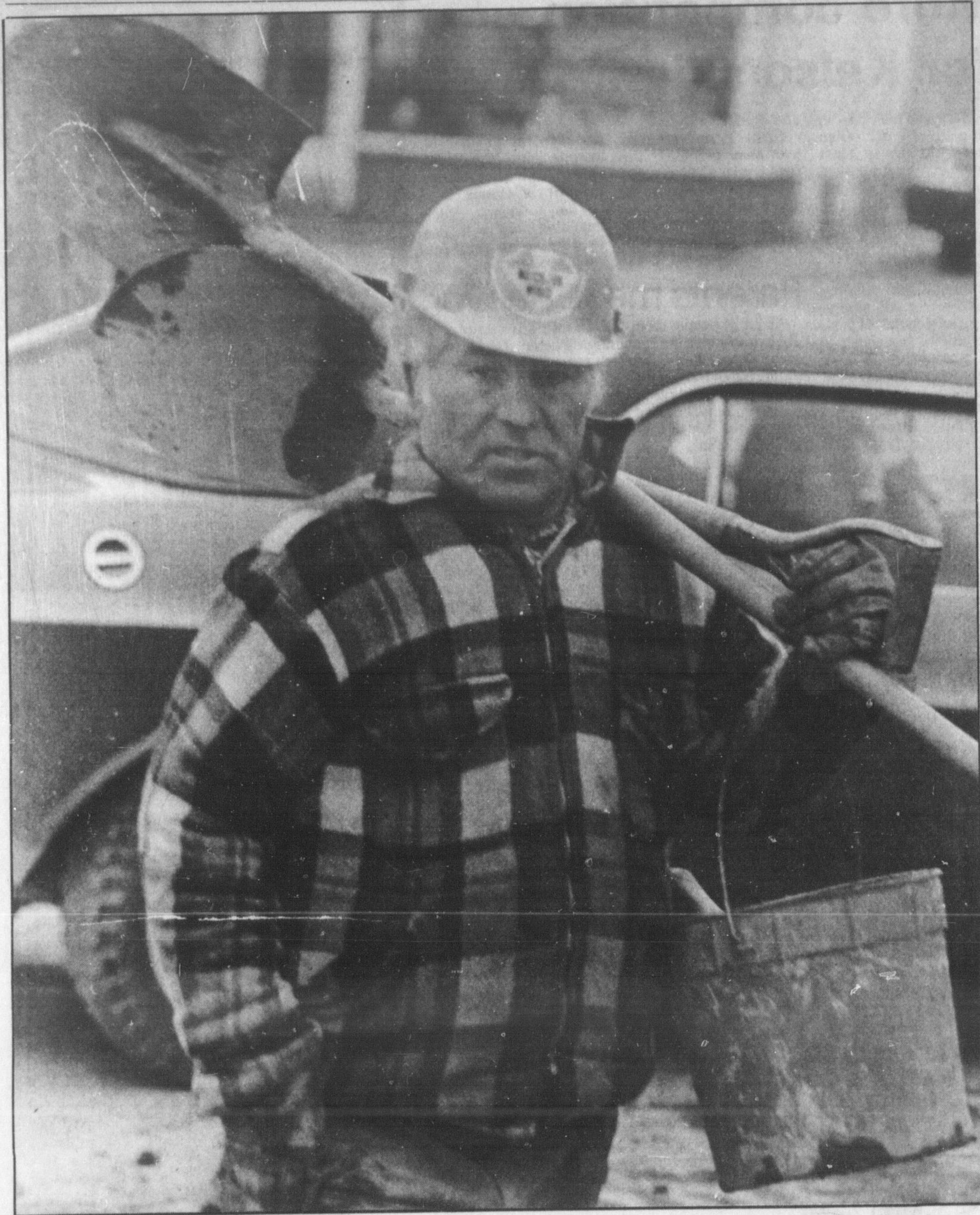
The cool weather makes outdoor work a little more difficult. Here, a construction worker, at the overpass at Ontario and Main bundles up for the job.
