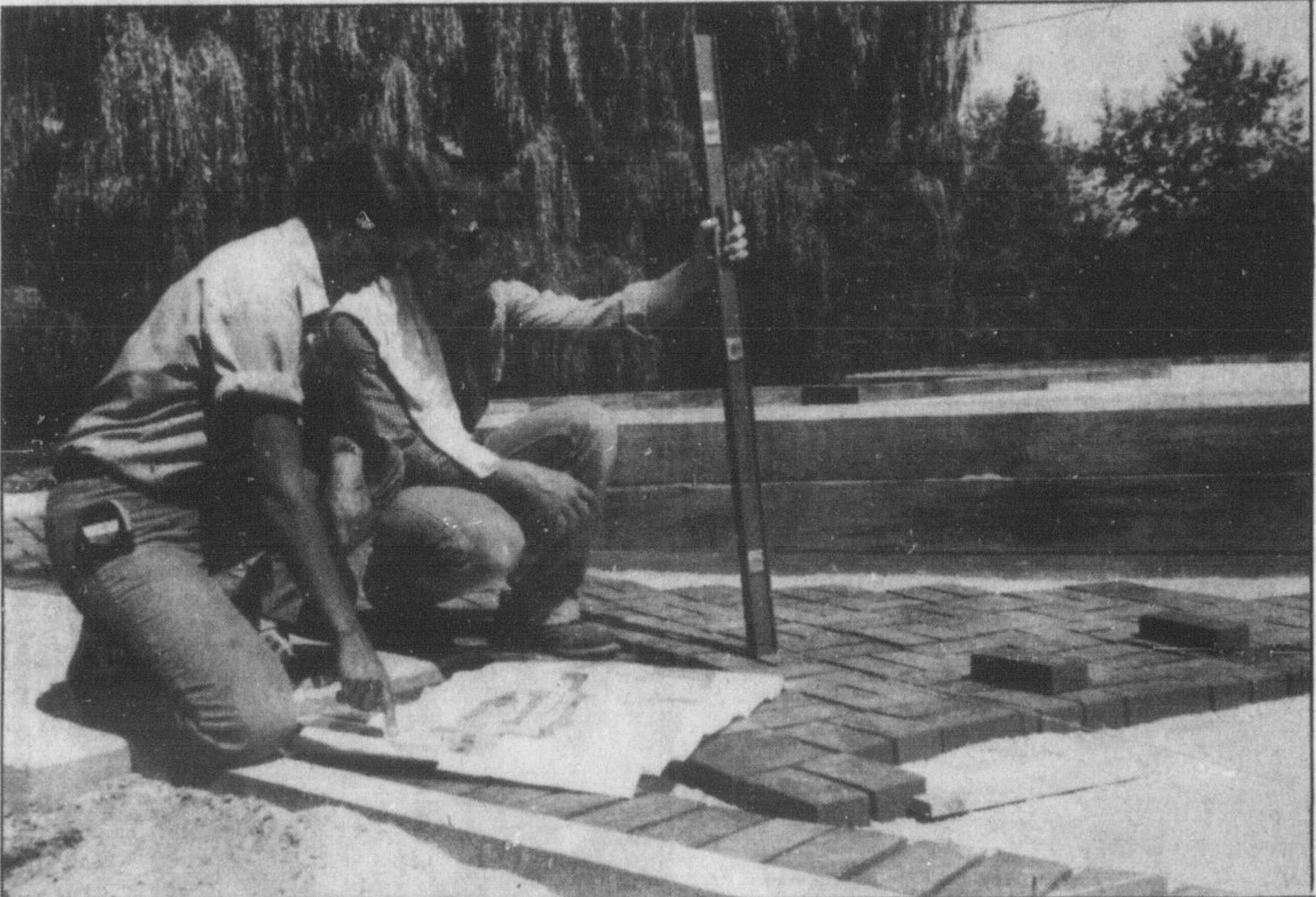
Checking the plans. Lisa Hageman, project supervisor and Stanley Luciw, a member of the construction team, examine the plans for an 18-hole mini-golf course, at Kelso Conservation Area. The project is expected to be completed within the next week.
