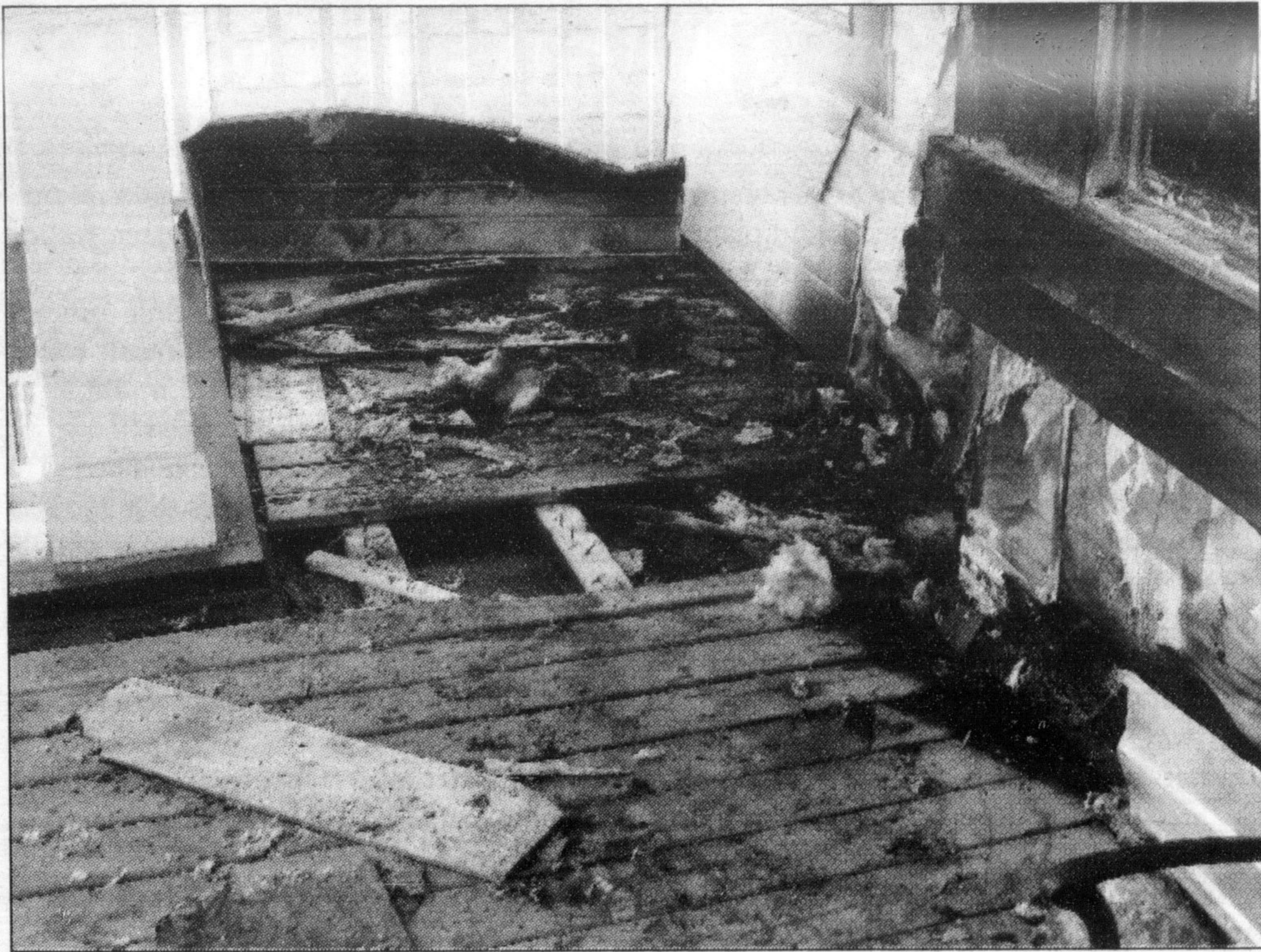
Fire caused extensive damage to the balcony of a Moreau Lane home. Firefighters believe the blaze started from the sun heating up dried peat moss in a flower pot.
