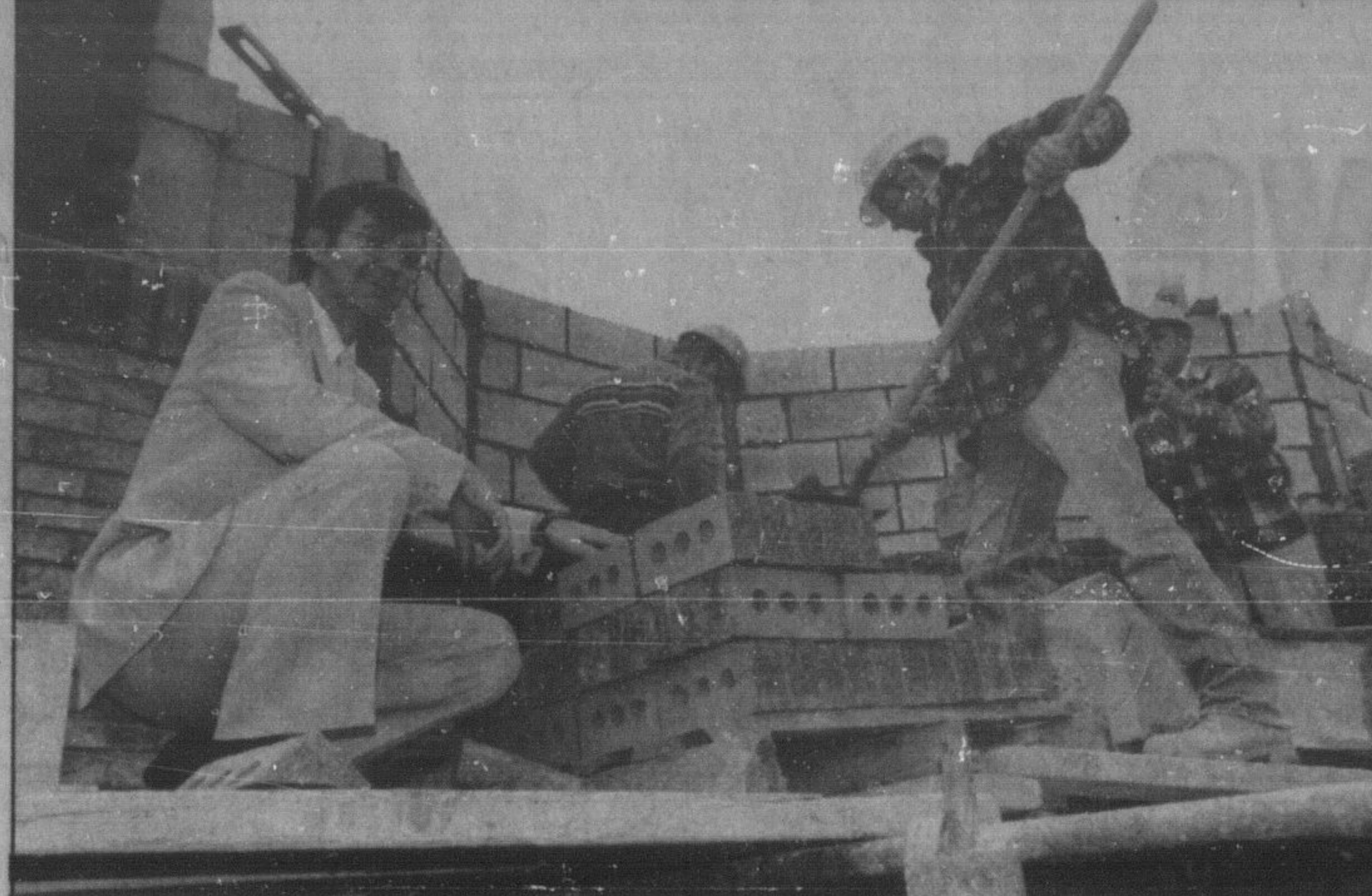
E.W. Foster Public School is progressing on schedule and principal Ed Wiens was on hand recently to take in some of the construction activity. An in the schools report on E.W. Foster appears on page D4 of today's newspaper.
