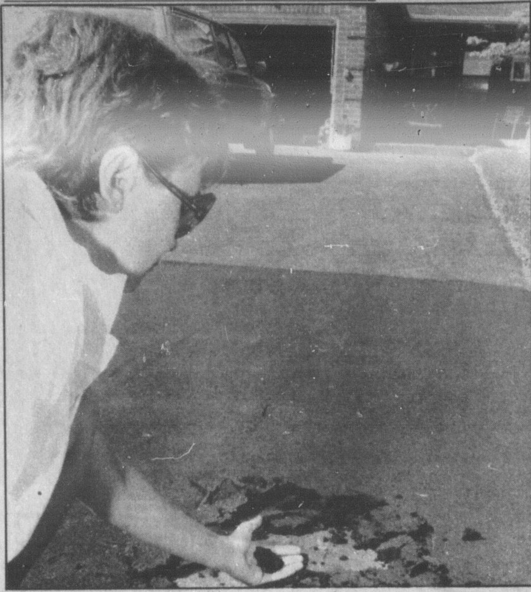
Alynne Huebsch, of Vanier Dr., illustrates a "repair" job done on the driveway of her new home by Silver Paving Co. Ltd. Several residents of Bronte Meadows and Timberlea developments have been expressing anger at what they feel is standard work carried out by the contractor.
