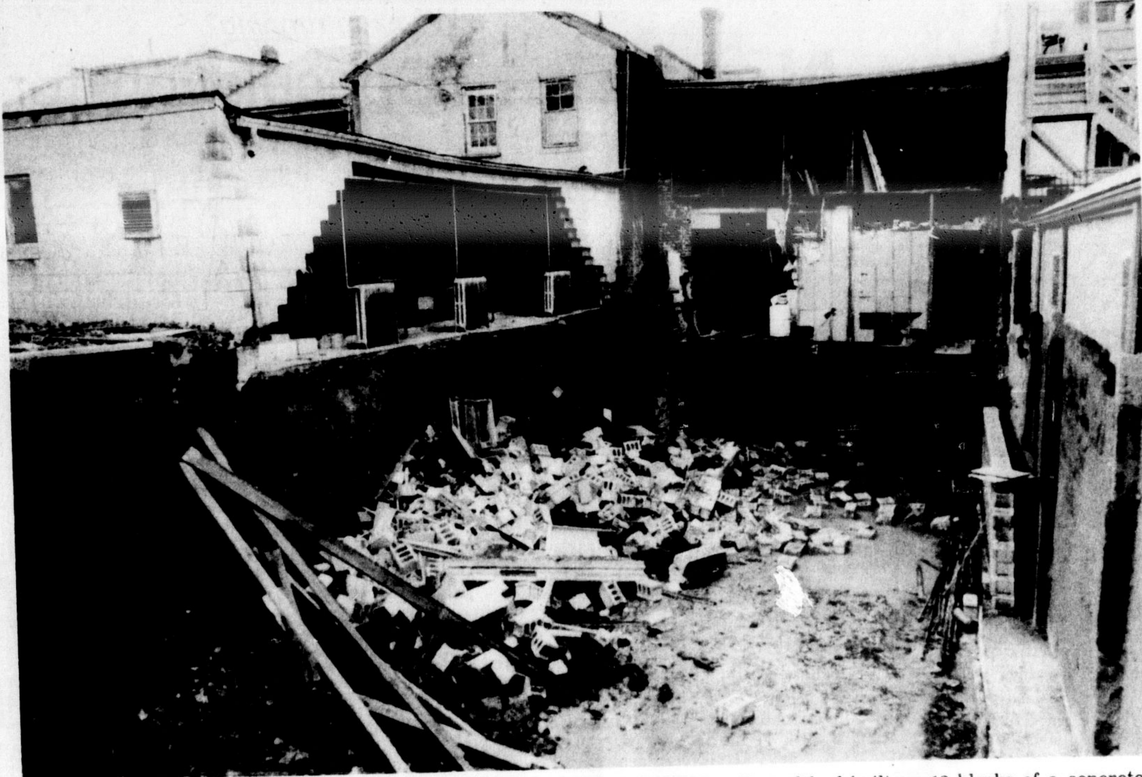
THE WALLS CAME TUMBLING DOWN: The side wall of Jim's Billiards on Main St. fell into an excavation at noon hour Saturday, after weekend rains weakened the ground beneath the concrete floor supporting the rear section of the pool hall. Neighboring store owner Ben Crisci had excavated a 20 foot hole beside the pool hall, to extend his stores south
