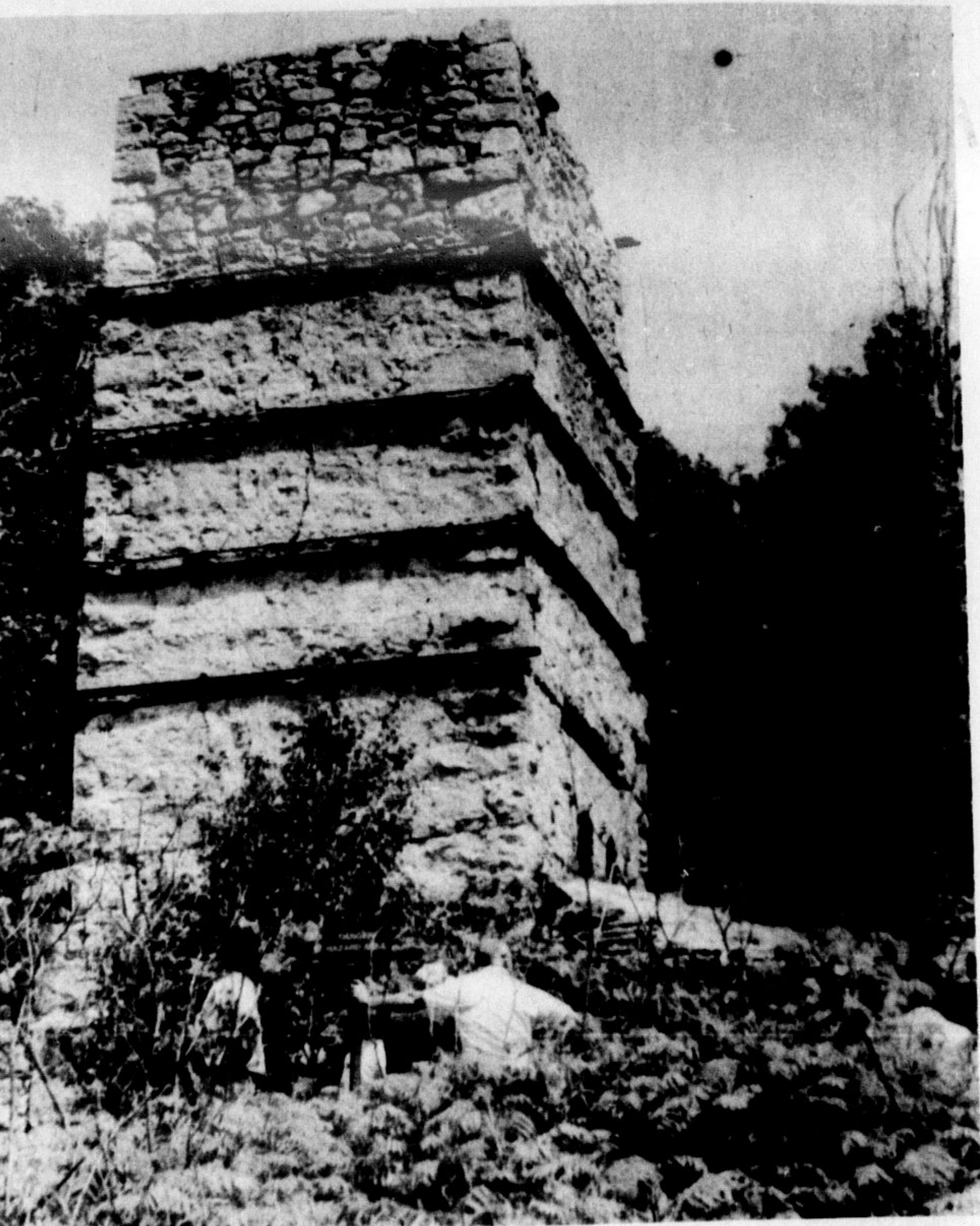
A PUBLIC HAZARD in their current state of disrepair, historic lime kilns at Kelso may be demolished unless funds can be found to reconstruct them. Besides the one shown here, there are two others, but one is already in ruins. The Christie Kilns were in use from 1880 to 1929.
