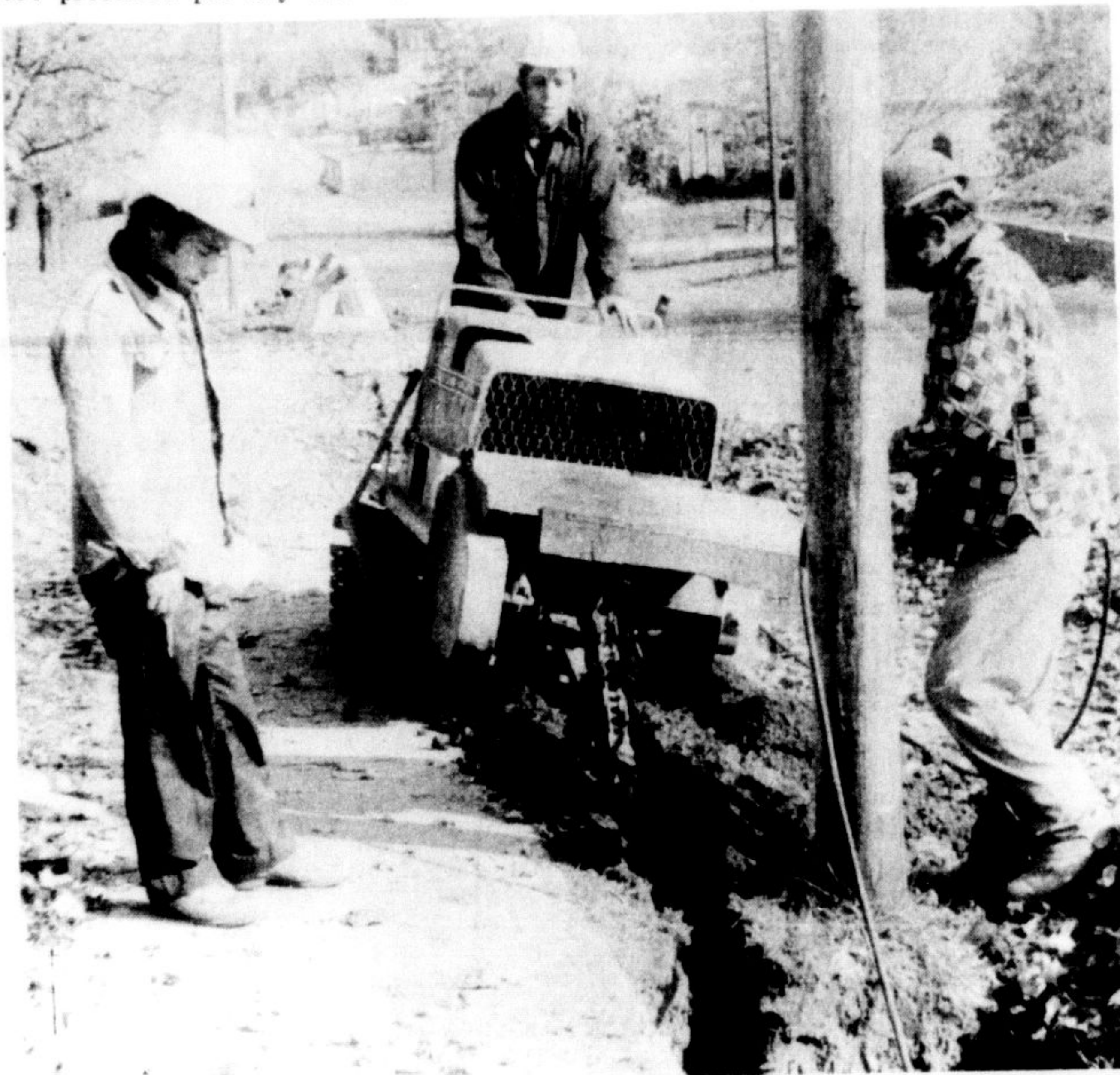
BELL CANADA EMPLOYEES were hard at work these past few weeks finishing laying telephone cable on parts of Martin St. and Woodward Ave. From left, Eddie Bravo, Sabino Conceicao, and Gabriel Coroa dig up the real estate on Woodward Ave. preparatory to the laying of the cable. The workers were scheduled to have finished the project yesterday.
