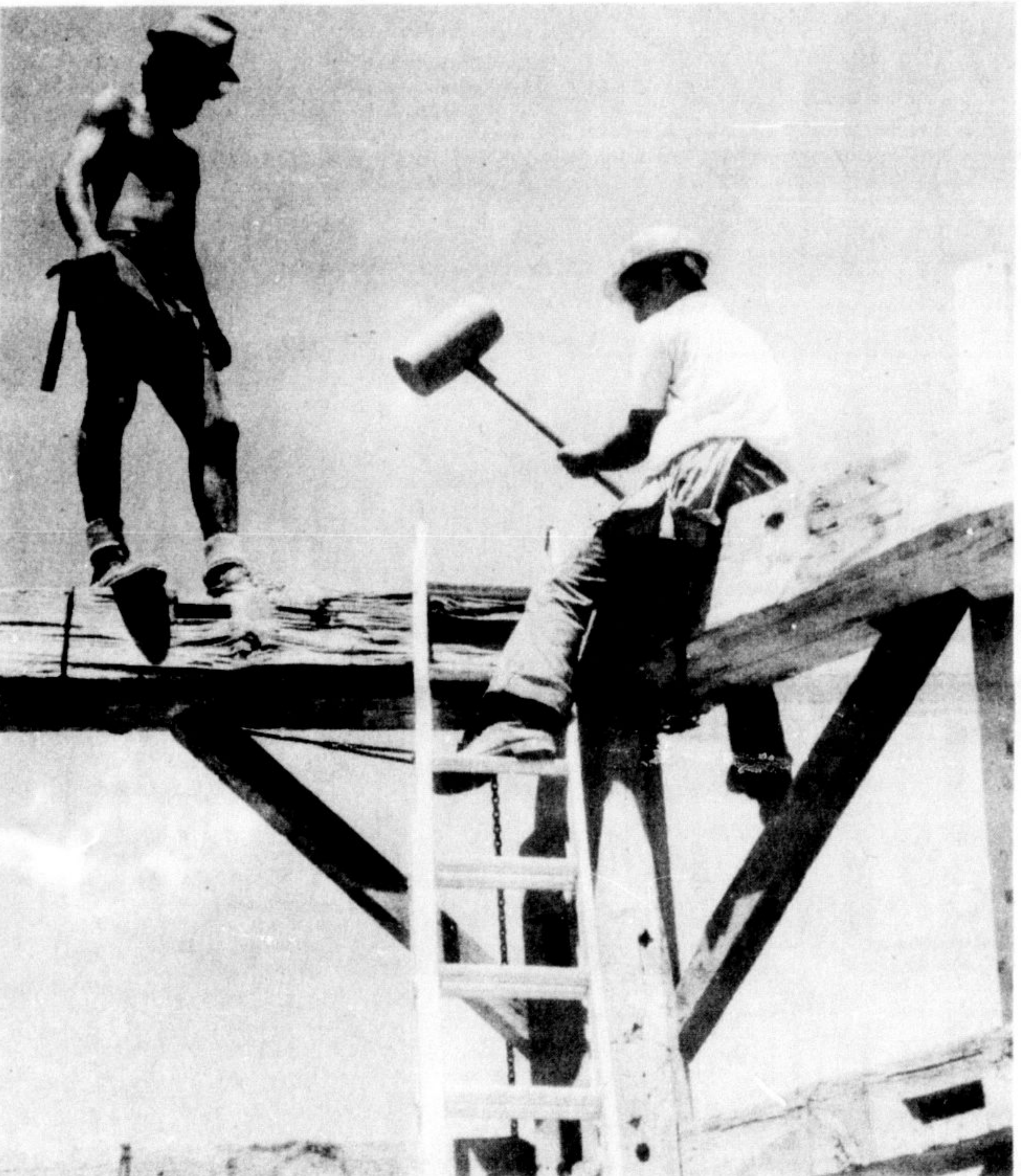
WIELDING THE BEADLE or persuader to hammer in pegs used in reconstruction of octagonal barn is John Graham of Guelph, while Scott Murray of Owen Sound stands by, ready to assist. The barn is believed to date to 1885, although some of the timbers are even older.
