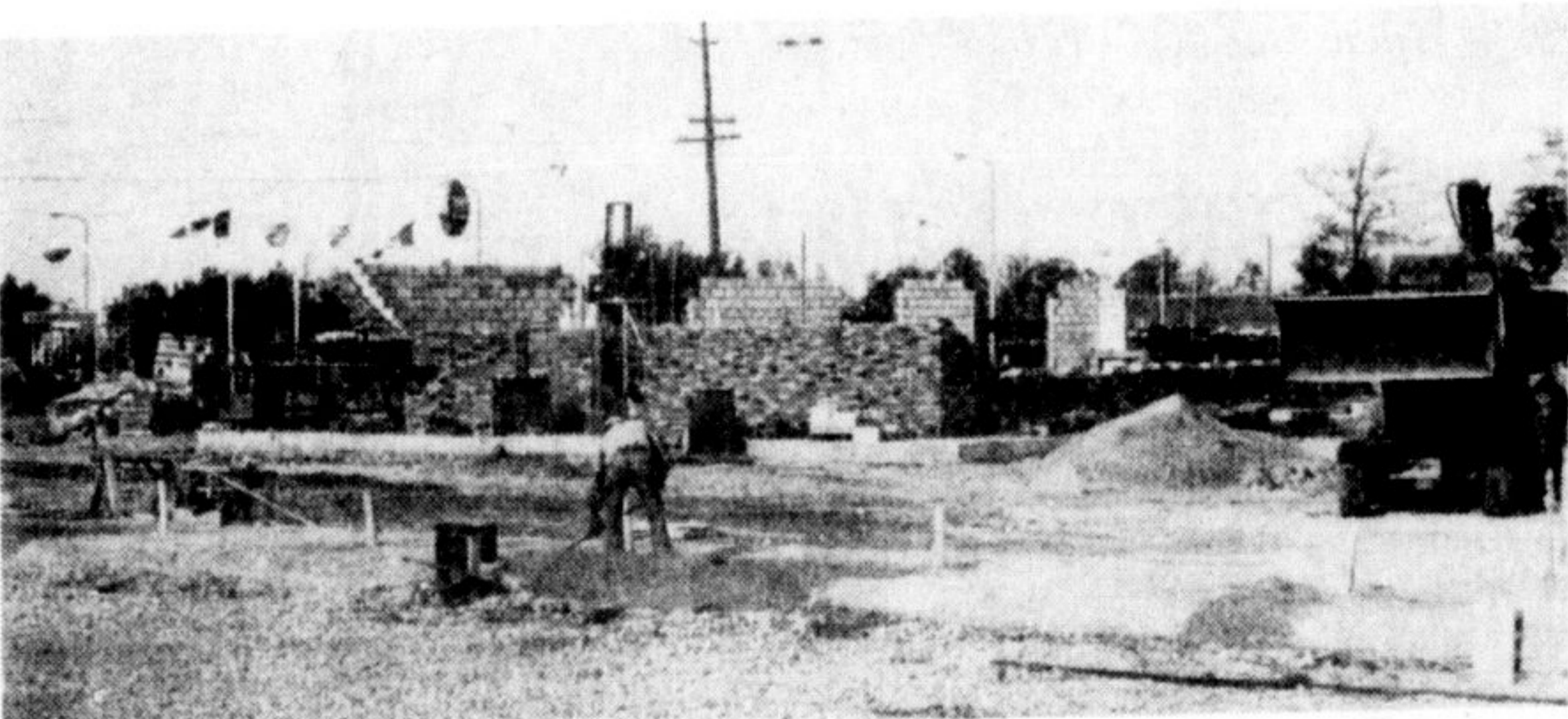
MacDonald's is coming to Milton soon, and workmen are erecting walls at the new $100,000 building on Highway 25 just north of Canadian Tire and next to North End Datsun. The restaurant is to be an eat-in or take-out facility.
