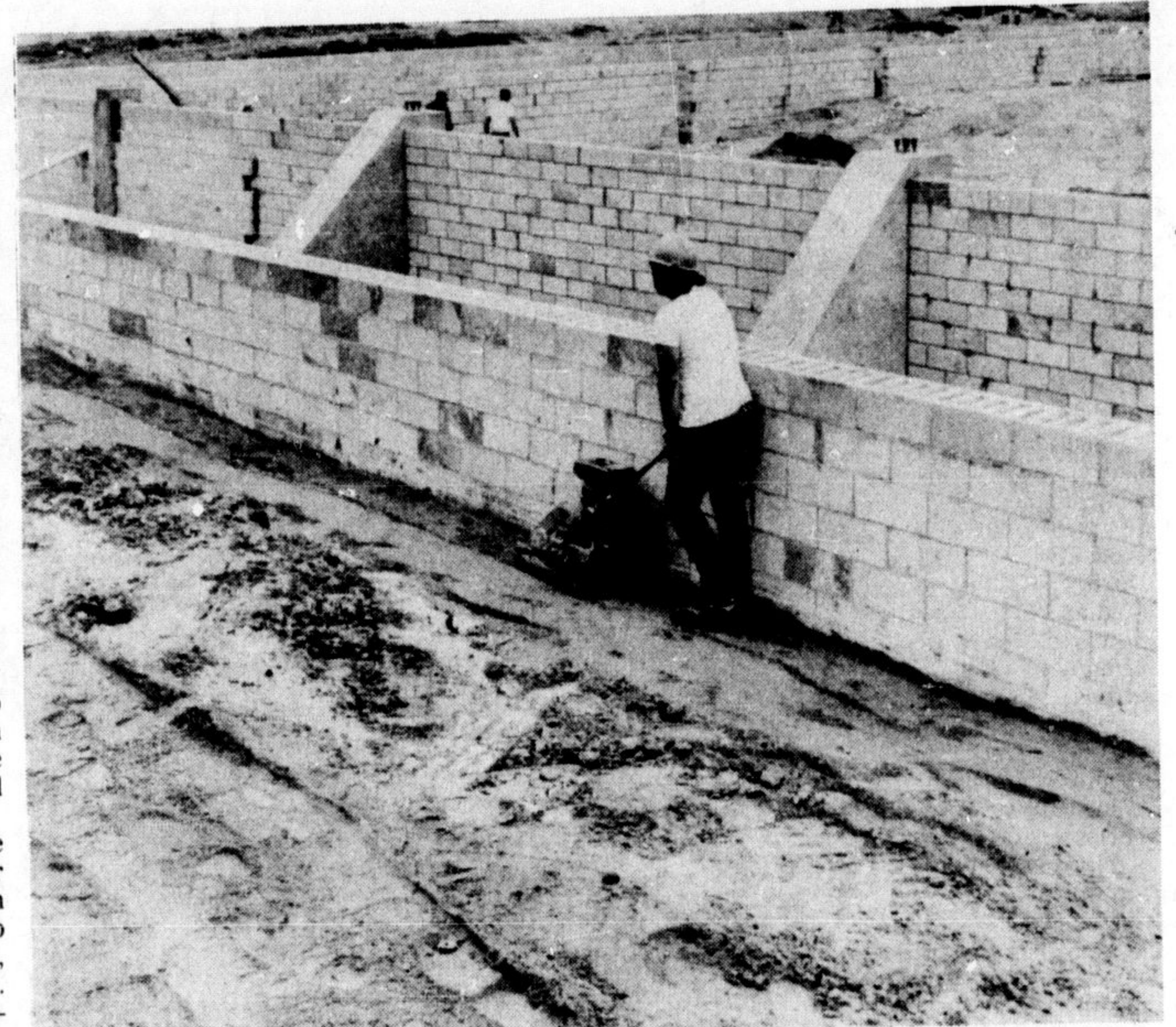
TO STRENGTHEN THE WEAK soil conditions, a worker pounds down sand beside the concrete block foundations of the new community centre. The steel section of the arena is expected to be put together beginning this week.
