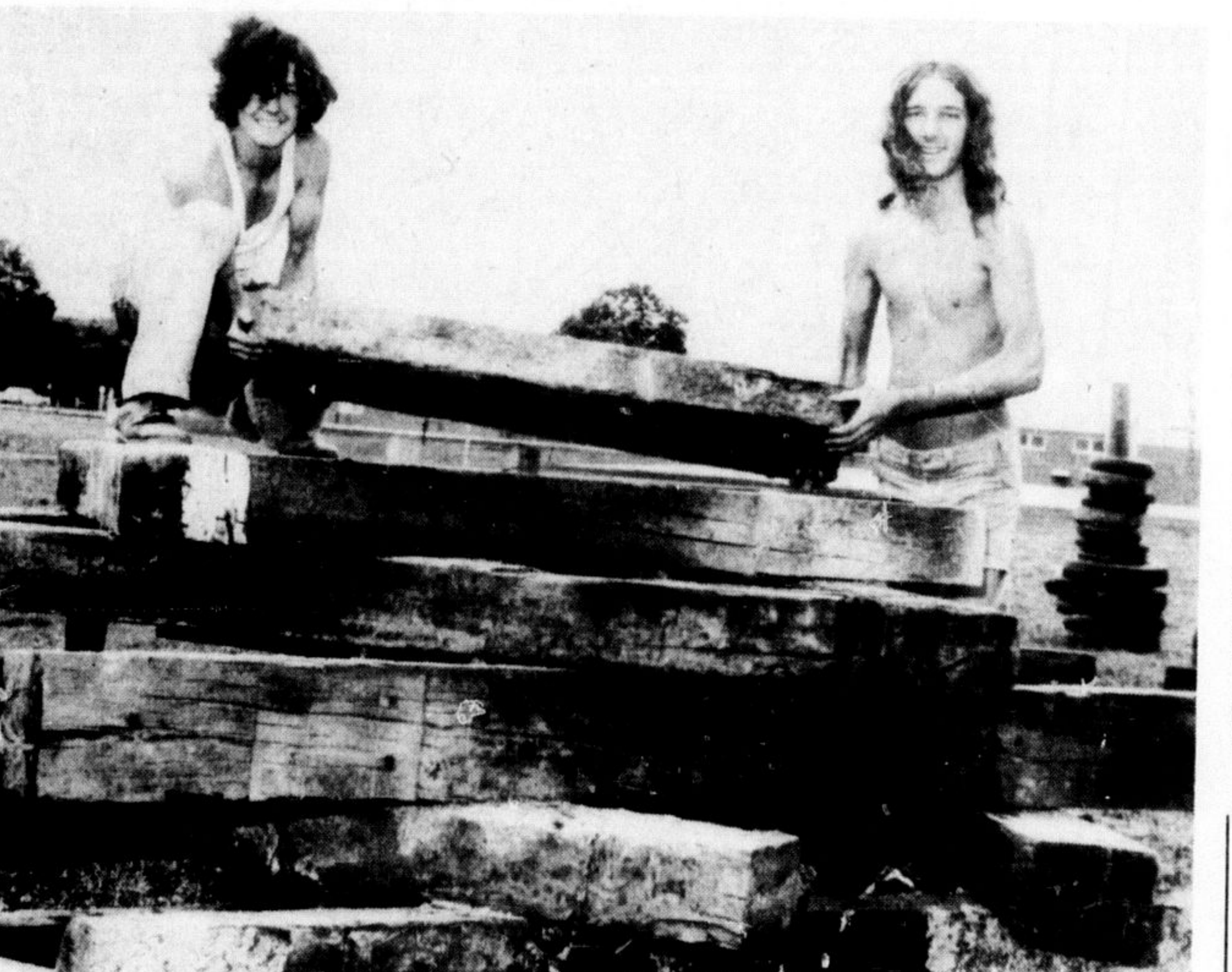
OFY WORKERS Chris Deschene and Graham Bell lift a beam into place as work on a pyramid or climbing apparatus nears completion. The pyramid is one of several innovative playthings that help make up the creative playground at Pineview School.
