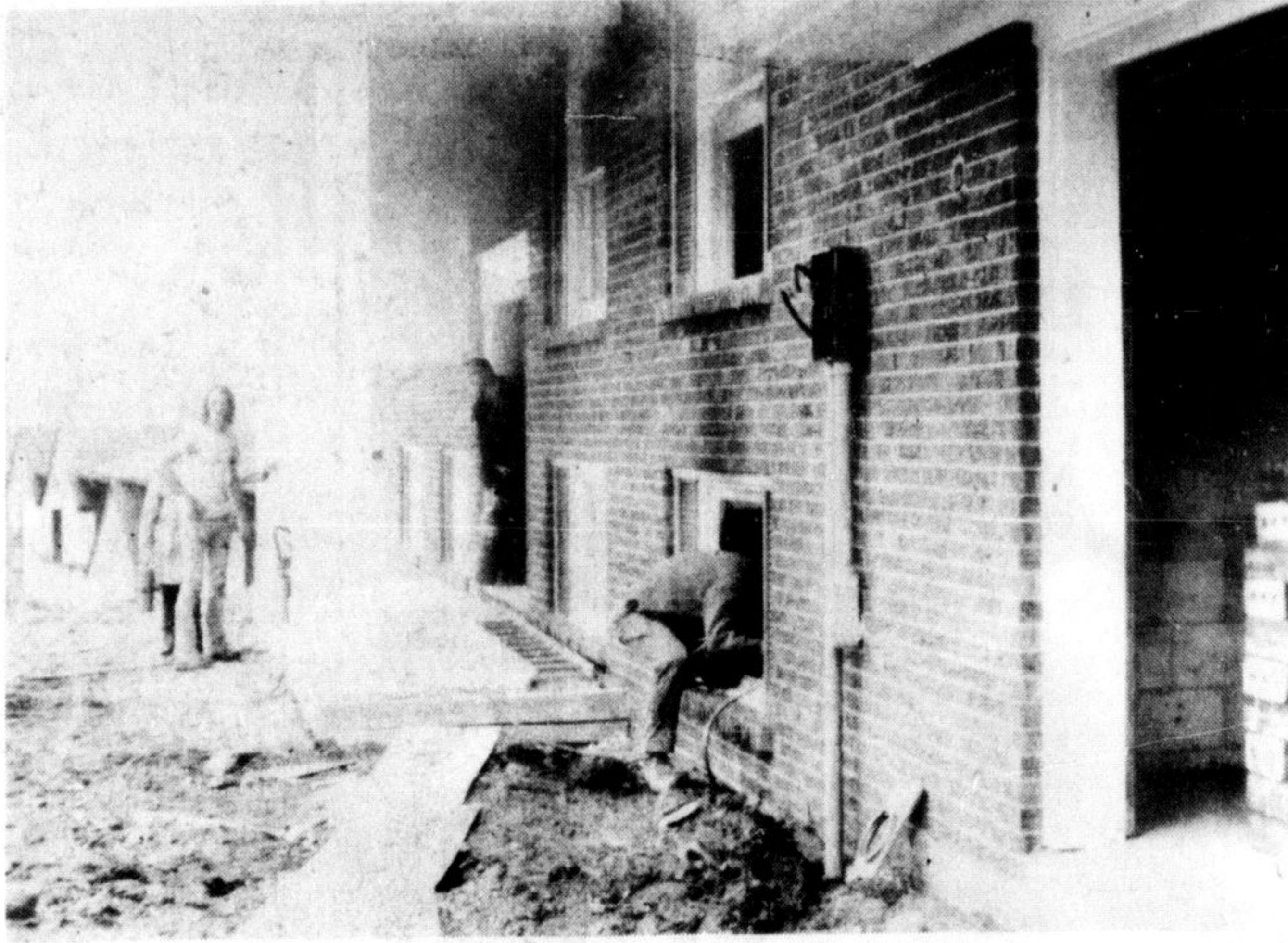
A HOUSE UNDER CONSTRUCTION in Campbellville suffered $5-6,000 damage Monday when fire broke out in the basement wiring. Some joists were burned and the home filled with smoke. Firefighters blamed a malfunction in the electrical wiring. The home is located in the Campbell Heights subdivision.
