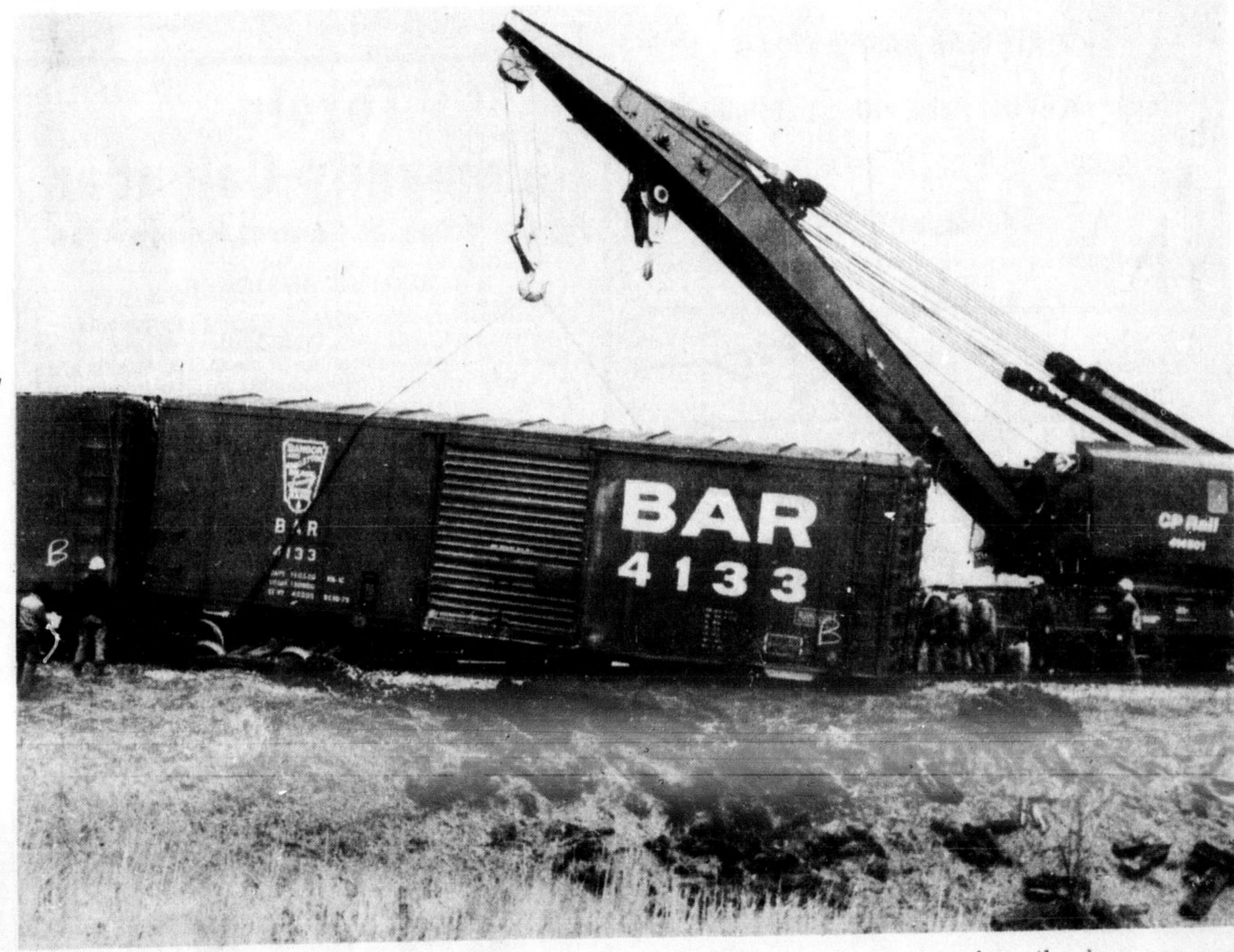
REPAIRING THE DAMAGE following the derailment of a box car on the Canadian Pacific Tracks between the Steeles Ave. and Bronte St. crossings Friday morning is a team of CP trouble shooters. The repair crew was roused from their beds before seven a.m. when the box car was jarrred from its wheels, left the tracks and plowed into the sod of the embankment. A crane (top) was needed to lift the car back onto the tracks. (Photo by D. Pink)
