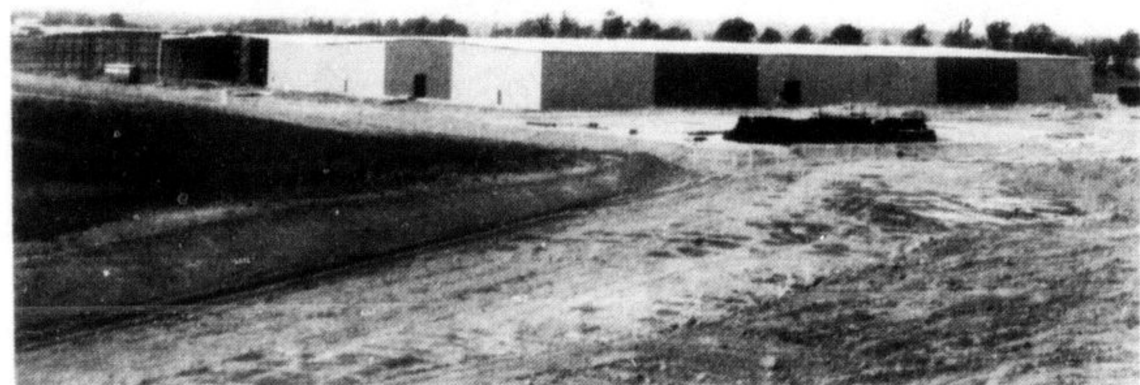
The new Consumers Glass distribution centre is taking shape as the webs of steel are enclosed at the Milton site. The plant will cover six acres of ground and the building is valued at $1,140,000. It is located on an 88 acre site off Chisholm Dr. at the junction of highways 25 and 401. The project is by far the largest industrial plant currently under construction and is a further mark of industrial progress in Milton.
