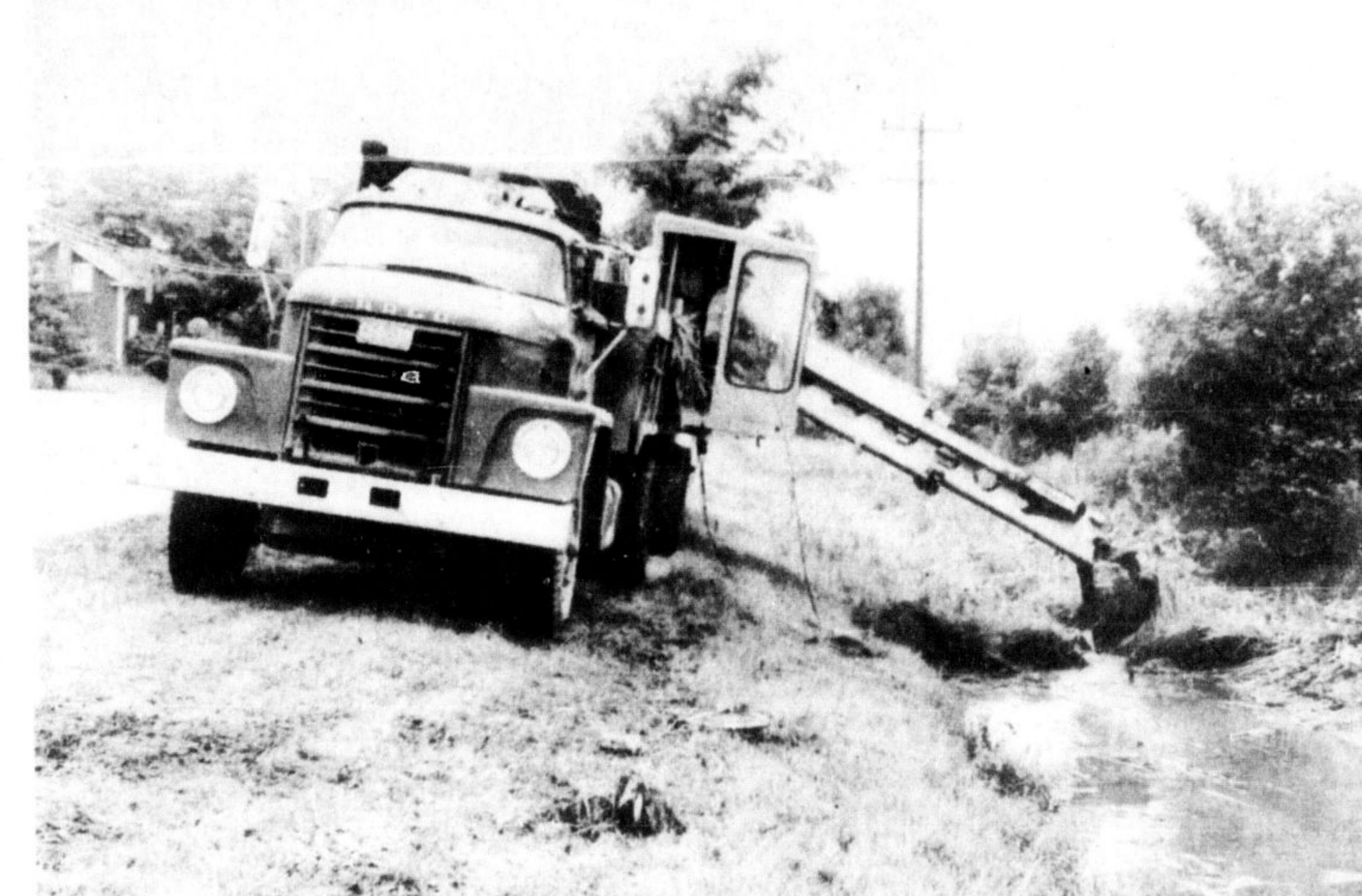
WATER FLOWED quickly once the Ontario St. Creek was dredged last week. Huge clumps of grass and earth that had been on the creek's bottom were
