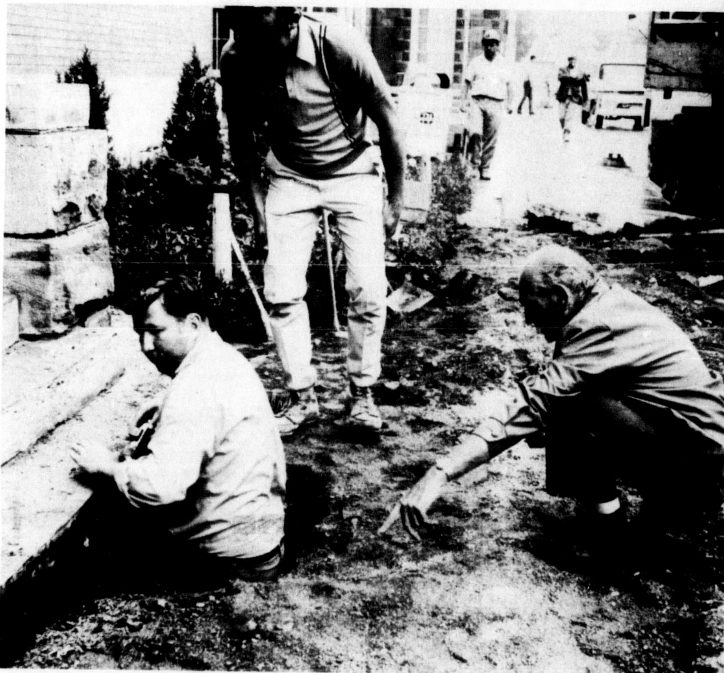
A MYSTERIOUS HOLE came to light one day last week when workmen were ripping up the sidewalk in front of Milton Post Office preparing to lay a new walk. The hole, about nine feet square and three feet deep, was discovered beneath the main front steps of the Post Office building. Nobody knows for sure how long it's been there, or why, although some oldtimers report the site was once a feed
