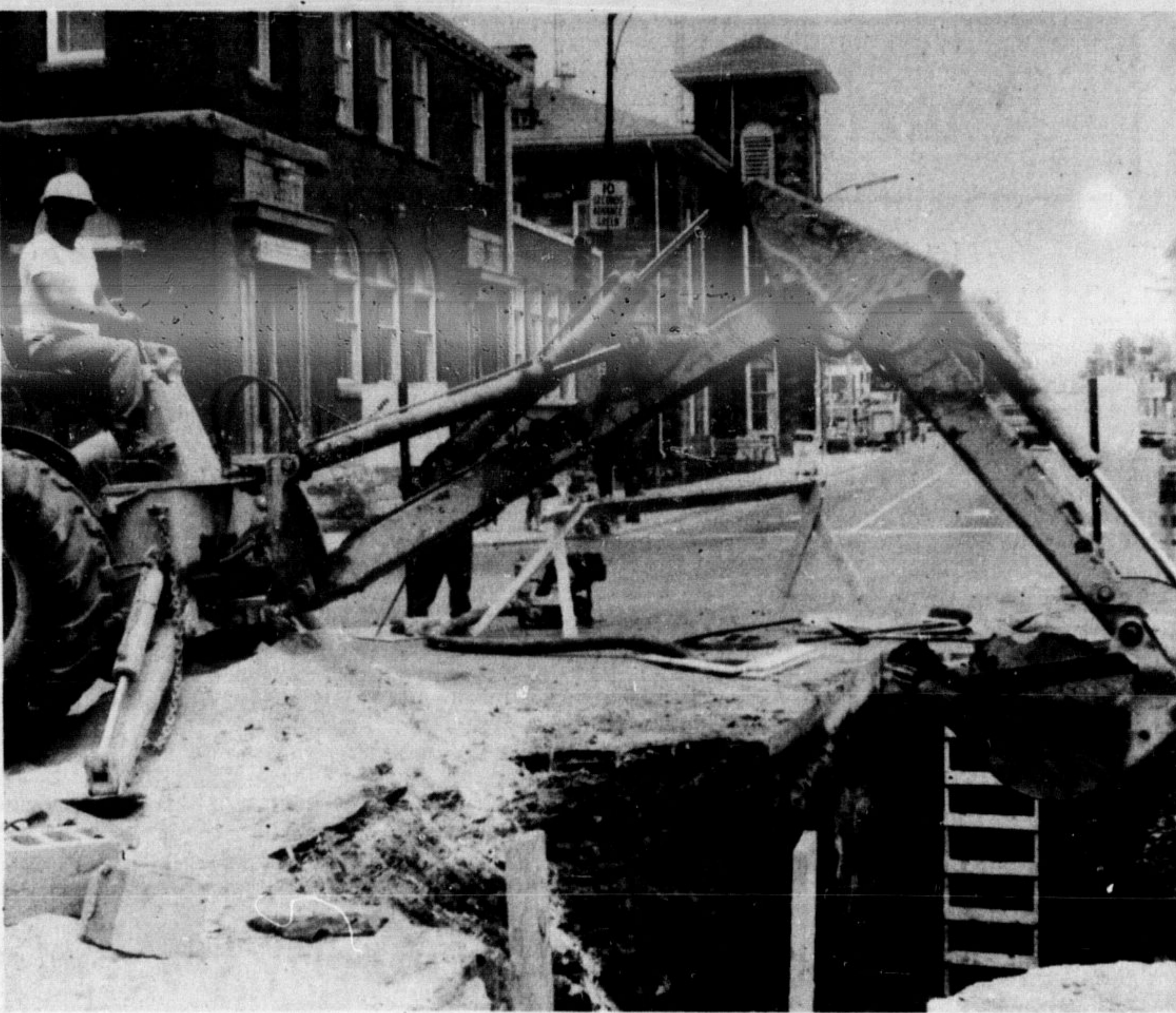
MAIN ST. RECONSTRUCTION is going ahead this week and workmen from Fermap Paving are still laying a 12 inch watermain up the north side of the street. The entire road between Martin and Bronte Sts. will be reconstructed this summer. Monday, they had a large hole dug at the Main-Martin corner and a machine is shown at work there. (Photo by R. Downs)
