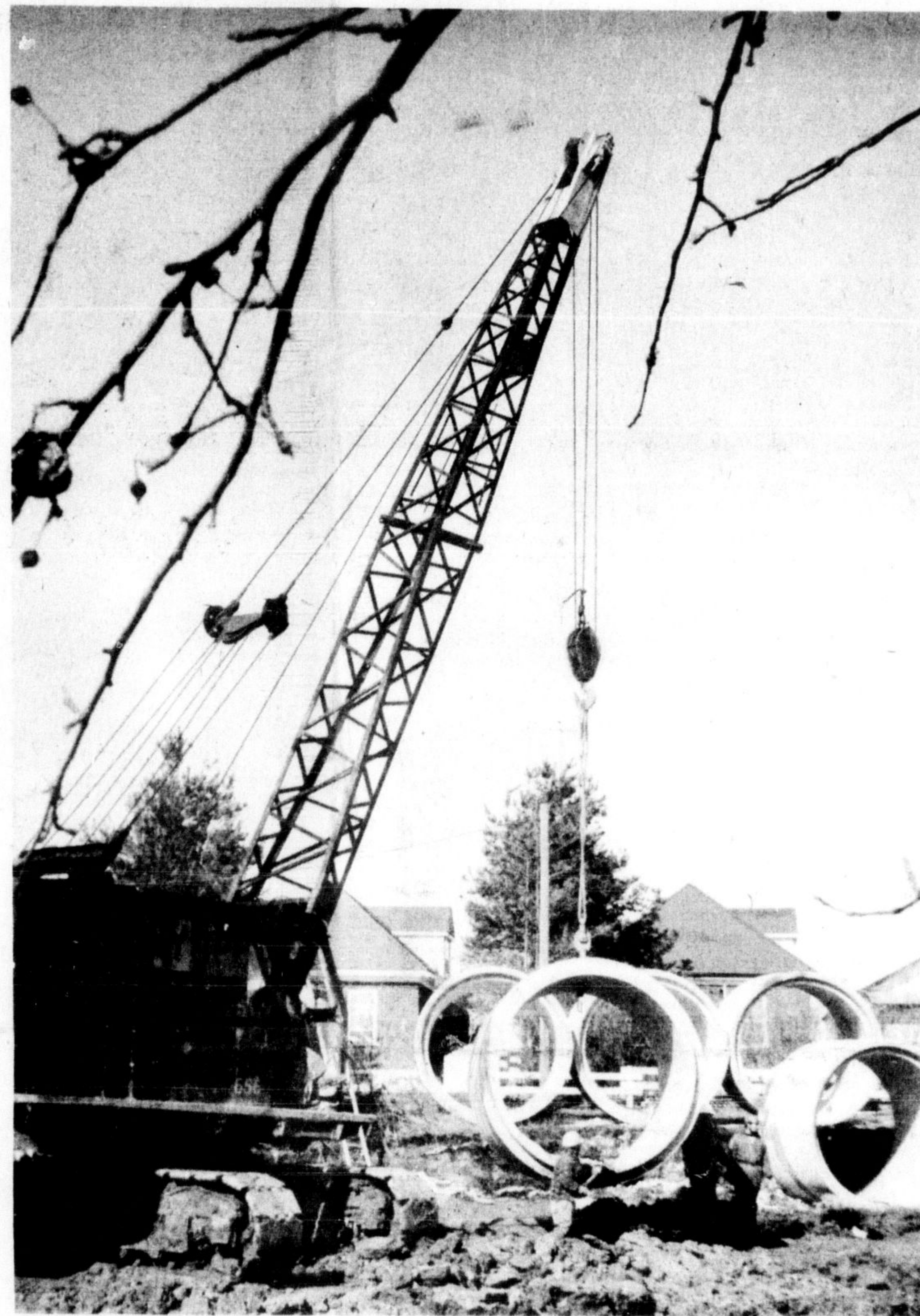
A LARGE TRUNK SEWER LINE is working its way across the north-east section of town as workmen from Wimpey Construction prepare for a 400-lot housing development east of Ontario St. Two lines are being laid, a two foot sanitary sewer plus an eight foot storm sewer, pictured here near the Court St. end. The firm is using a laser beam to ensure the line is laid as it was designed. —(Staff Photo)
