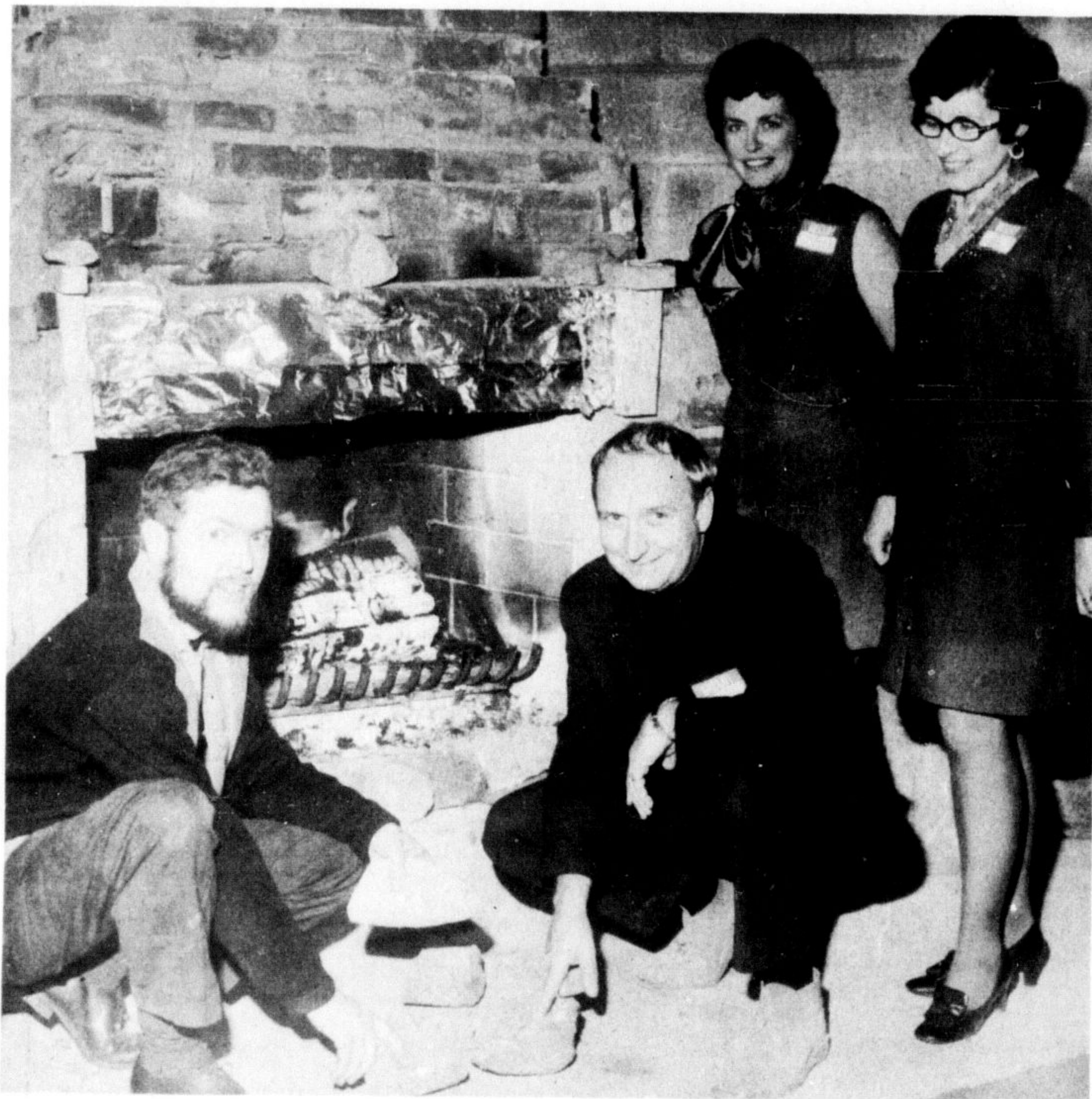
REAL NASSAGAWEYA STONE is being used for the stone face of this manmade fireplace at Bezek Centre, Second Line Nassagaweya. Piling stone for the fireplace while their wives look on are Rev. Bernard Warren and Bezek director Norman Hare. Mr. Warren and numerous volunteers have devoted their time
