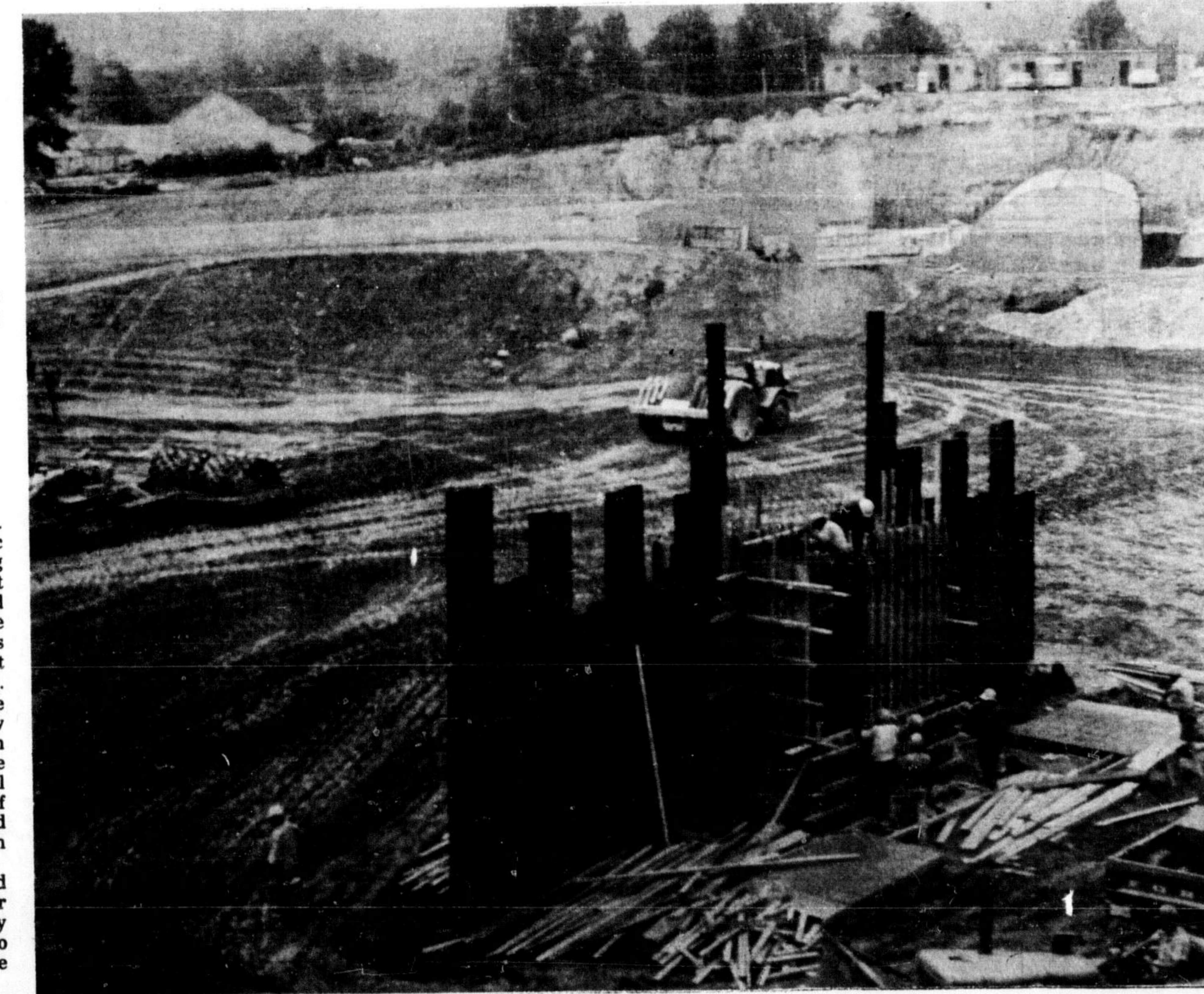
THE SCOTCH BLOCK DAM, a project that has been on the board since 1964 is coming along according to schedule according to BOT Construction spokesmen. BOT is the general contractor for the job.
