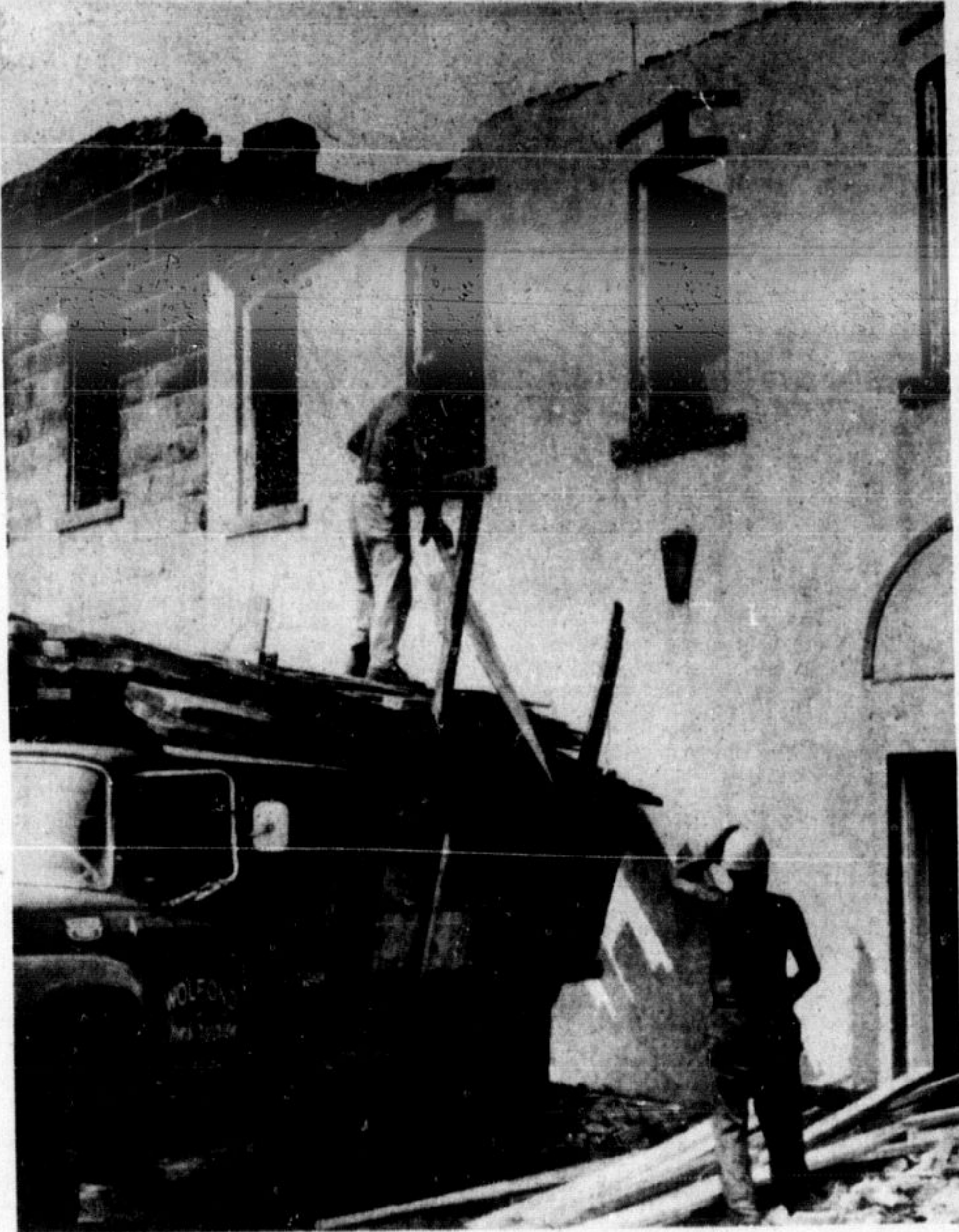
THE CENTURY OLD BUILDING at the corner of Main and Charles Sts. is slated for destruction and workmen were scheduled to begin tearing down the stone walls today (Wednesday). Employees of Wolfond Construction, Guelph have been stripping the building of all useable materials before knocking in the main structure. The building has recently been used as a bakery and music store—before that it was a funeral chapel and furniture store.—(Staff Photo)
