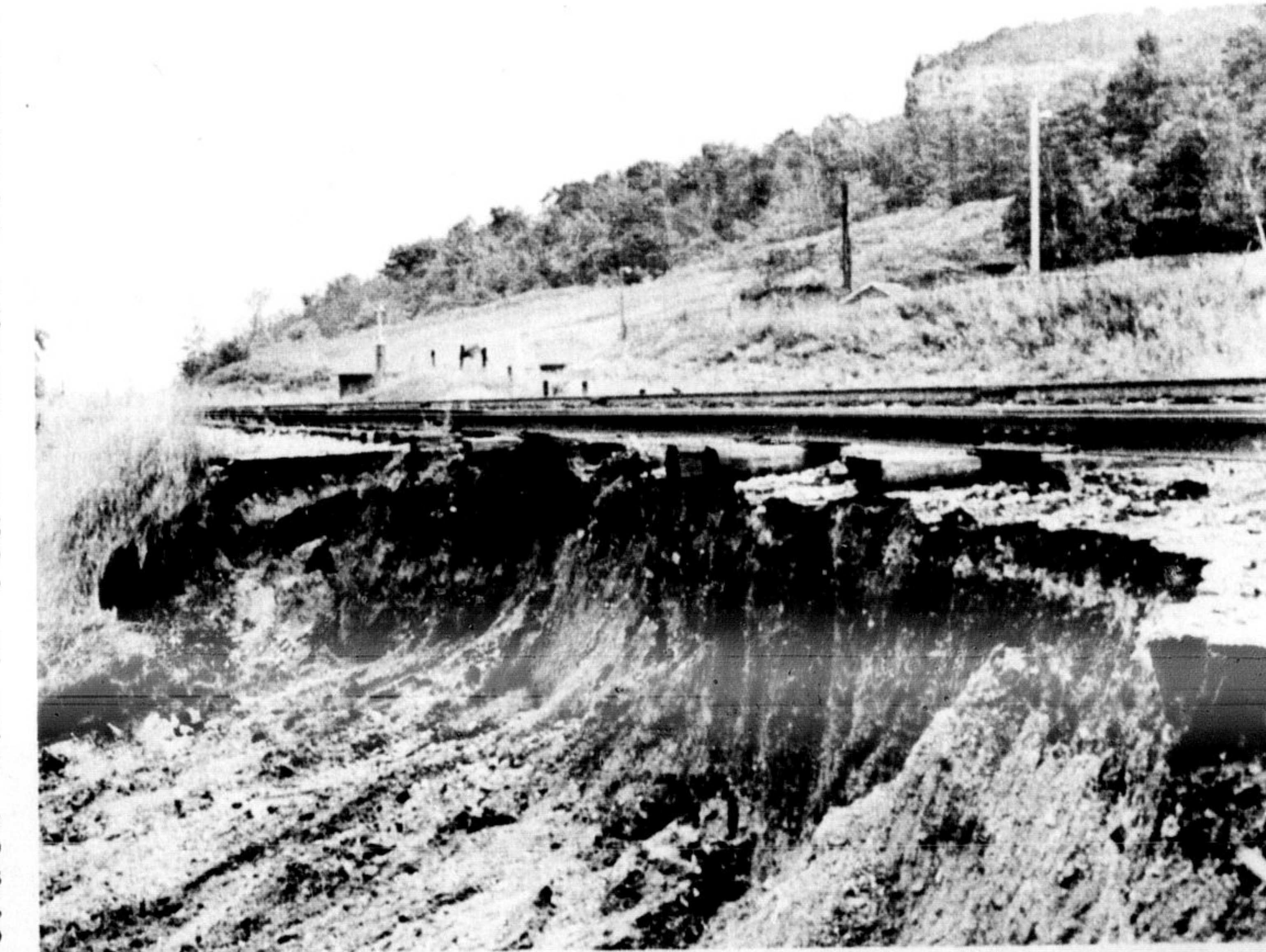
TORRENTS OF WATER washed the bank under a section of siding on the CPR main line at Kelso Saturday. A section of the main line bank 100 feet long was also eroded and had to be replaced Sunday morning after the four inch downpour hit the Milton area Saturday.—(Staff Photo)
