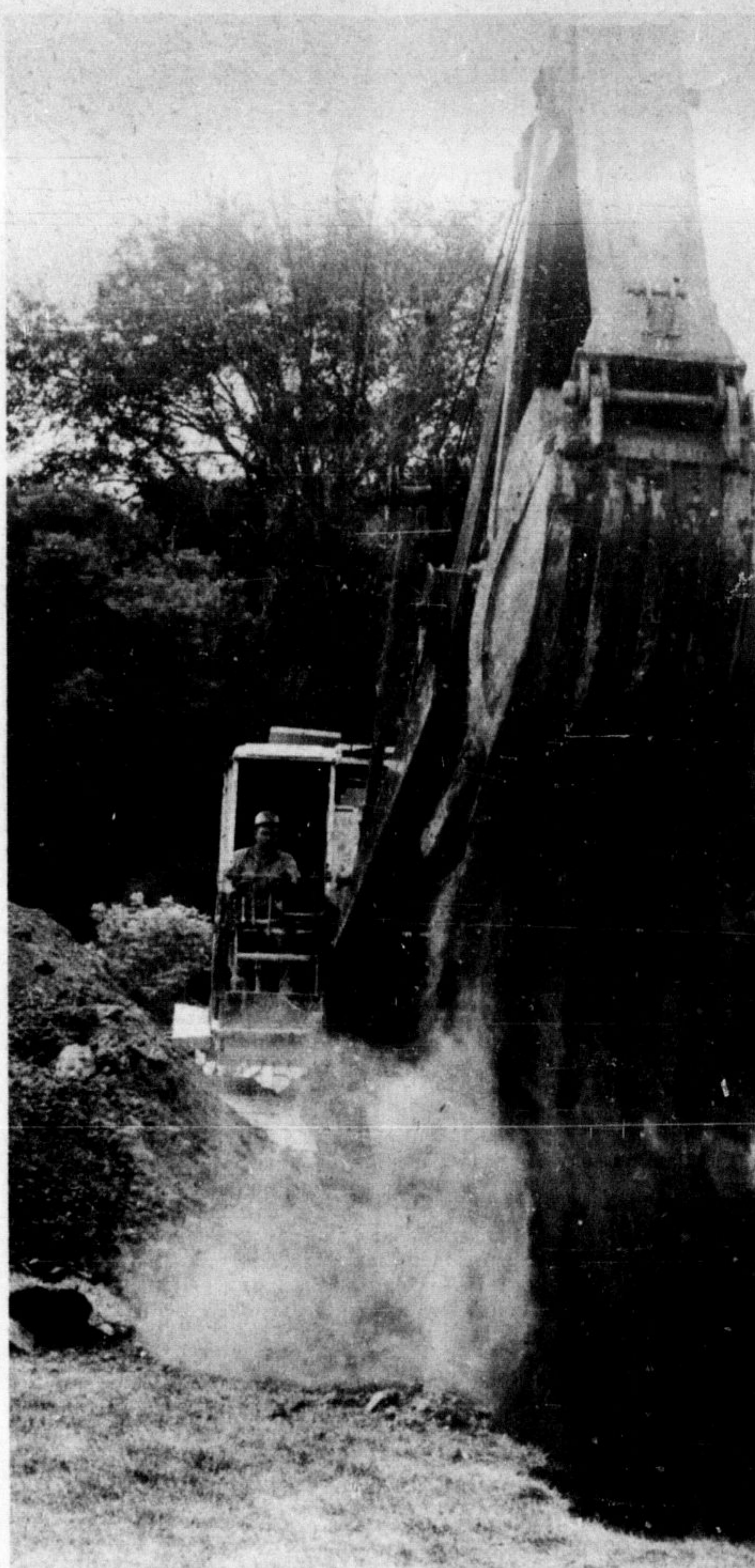
CONSTRUCTION BEGAN on the first phase of the trunk sewer at the Fulton Street plant Monday. It is hoped construction will be finished in November but there is a 30 week waiting period for some of the tanks. Eventually the pumping station at Woodward Street will be eliminated, but the first phase just goes as far as the Fulton-Oak St. corner. (Staff Photo)
