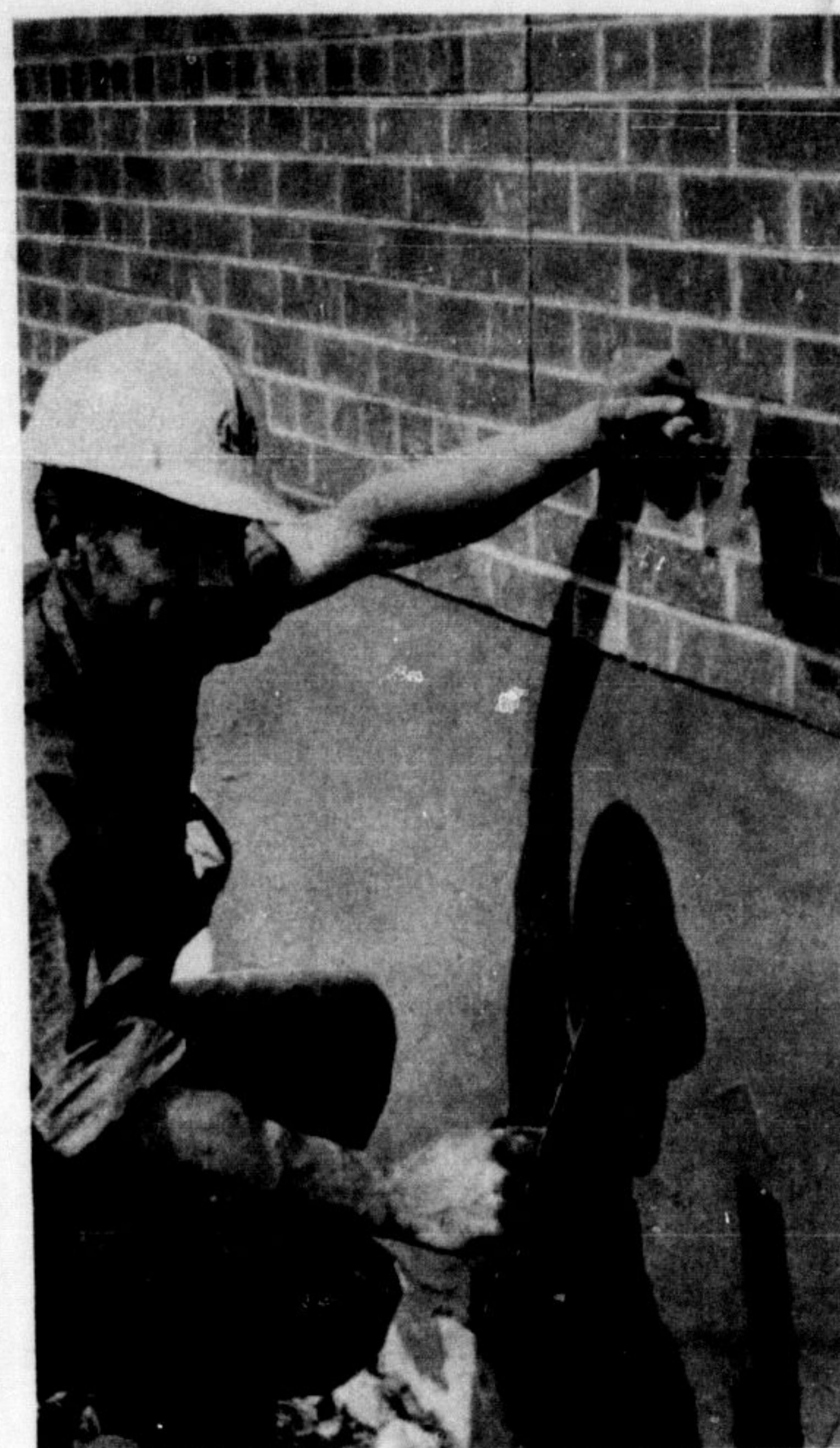
SOLID NEW WALLS TO CABLES causing problems, there's plenty of activity at the new M.D.H.S. addition. Here bricklayer foreman Werner Koveck smooths out the foundation while at right sub-contractor Edgar Howden
