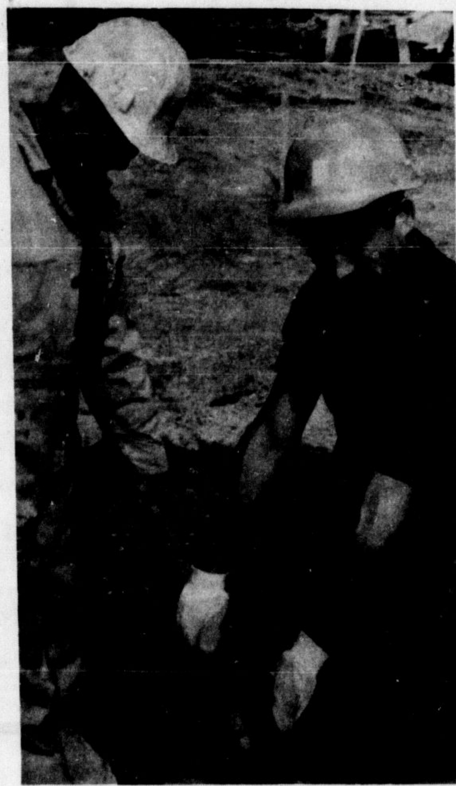
and Sam Campanes examine an unearthed telephone cable. Representatives of the high school board and the contractors meet approximately every three weeks to talk over progress of the construction. (Staff Photo)
