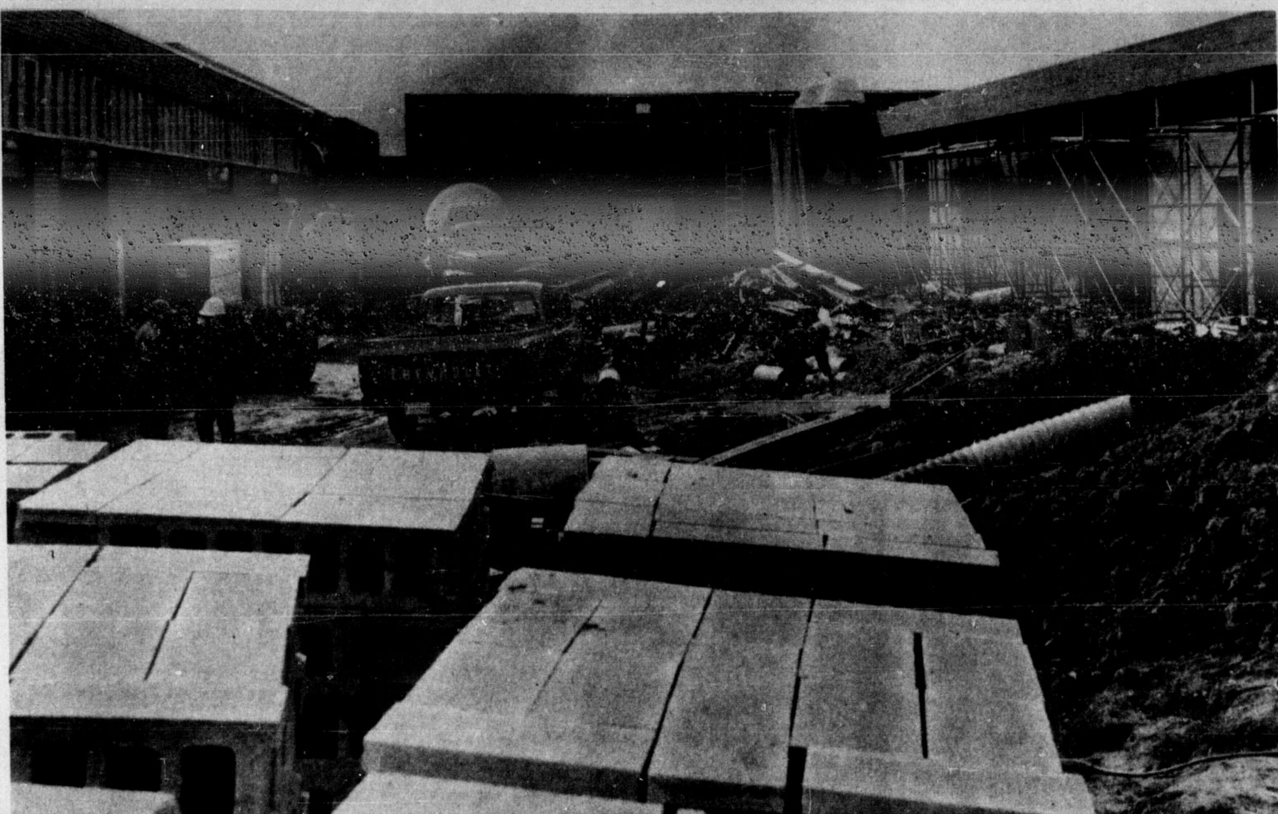
WHILE IT DOESN'T look it now, this will be four classrooms, a single (girls') gymnasium, change rooms, instructor's office and storage, a team room, science room, occupational training room, business office, practice room, electric typing room, accounting department, business machines, marketing and merchandising, workroom, commercial director's office and conference room at the end of four months. (Staff Photo)
