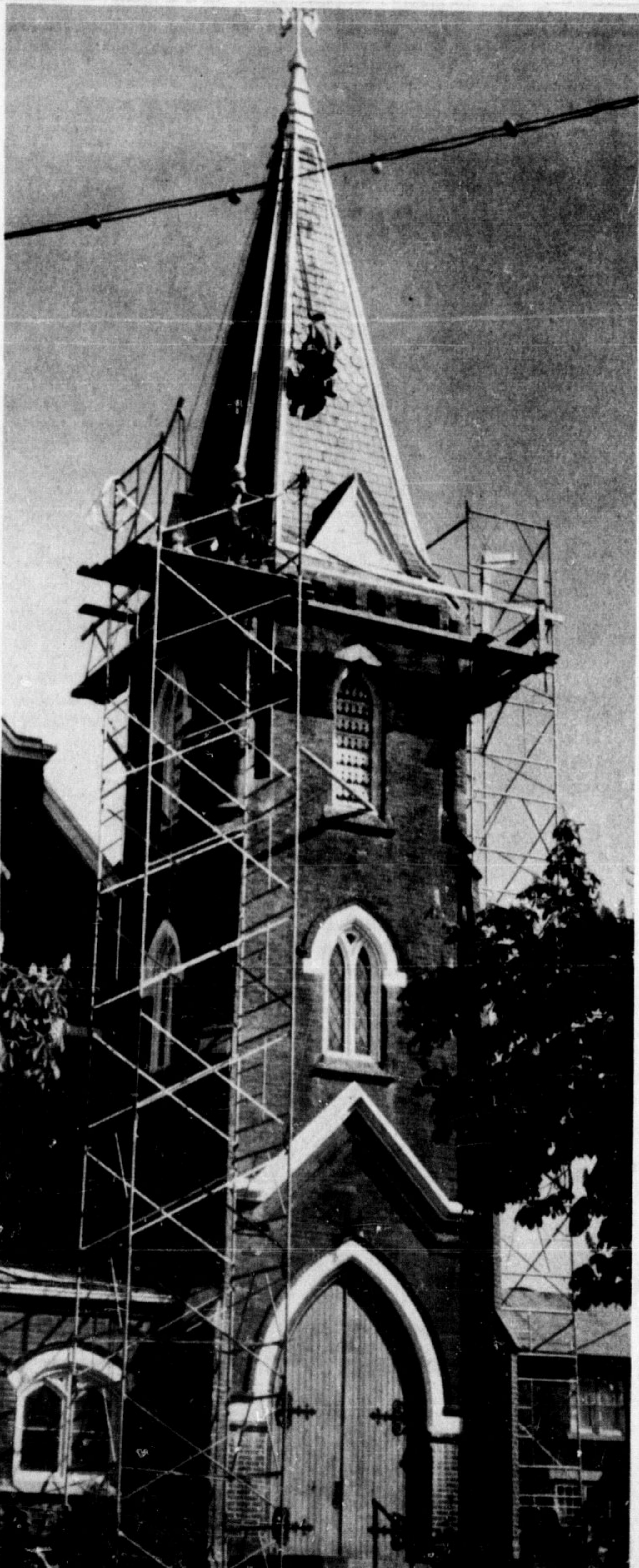
80 FEET ABOVE MAIN ST., steeplejacks are removing and repainting the old steeple on Knox Presbyterian Church. While they've won the admiration of a host of sidewalk superintendents for their aerial derring-do, the "jacks" have not yet been swamped with offers to trade places with anyone on the ground. They're not finished yet, but already the old tower is gleaming in the sun with its fresh coat of paint. (Staff Photo)
