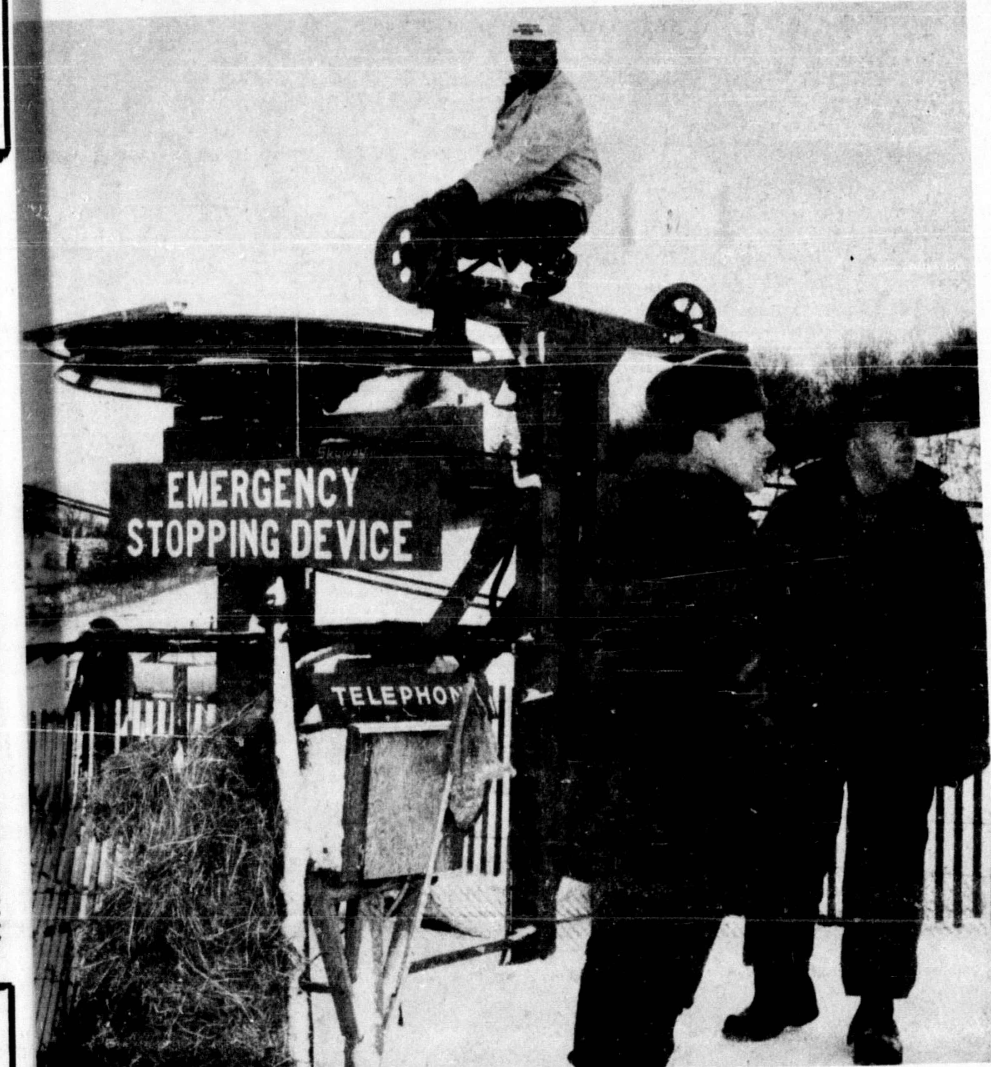
SKIING WAS DELAYED for two hours Saturday at Glen Eden Ski Club while workmen repaired the main cable. A crane was needed to lift the 1500 feet of cable back into place when the derailment occurred. Here Conservation Authority workman Slim Kangas makes an adjustment, while H.R.C.A. Field Officer Dave Murray looks on. (Staff Photo)
