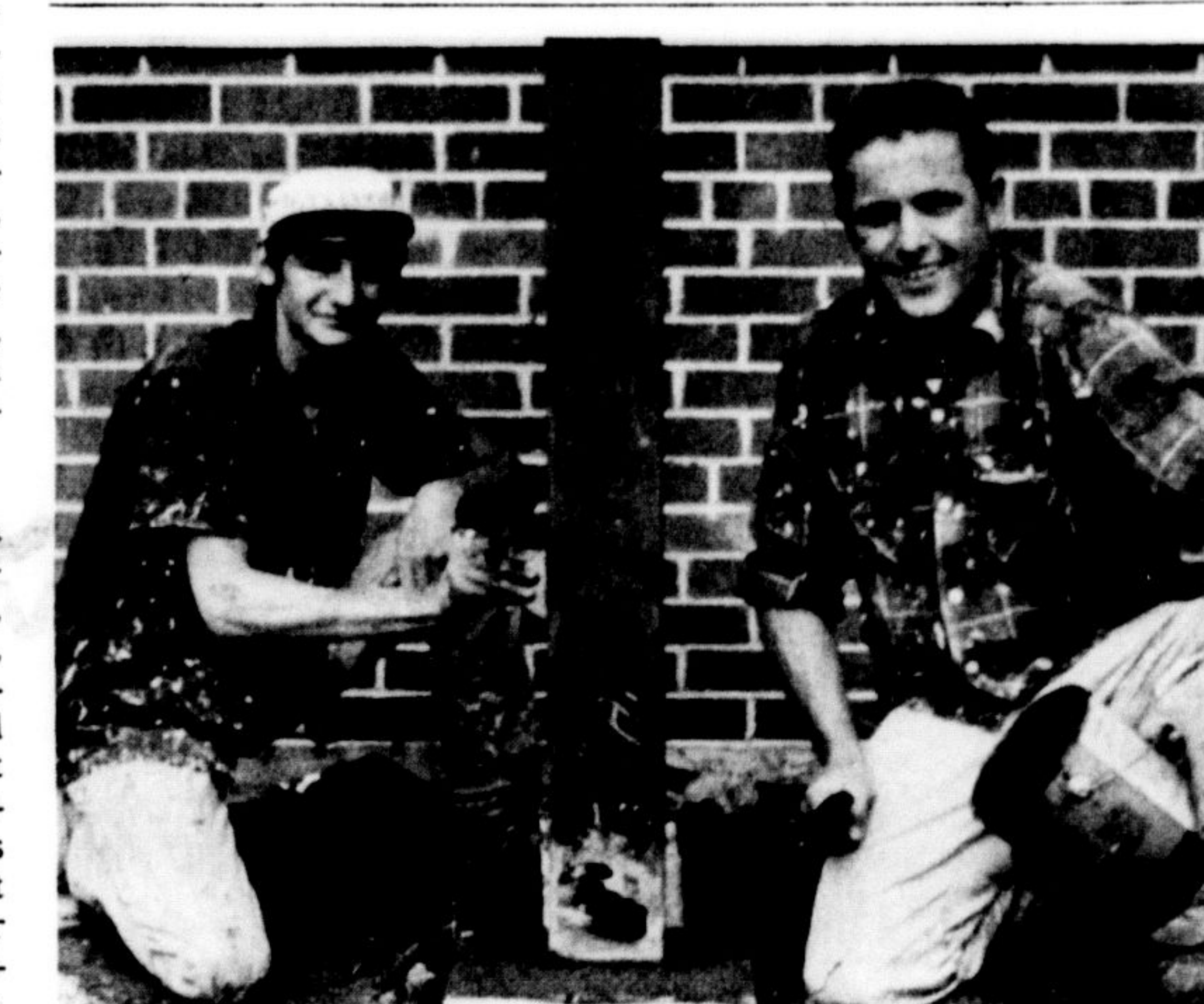
WORKMEN GIVE THE NEW WING at Brookville School the finishing touches. Joe Martini, left and John Gemin, both of Guelph, touch up poles outside the building. The $300,000 addition includes six classrooms plus a home economics room and industrial arts room and a library. Superintendent Mike Reidy of Battaglia Construction Company reports the building will be ready when school starts next Tuesday. (Staff Photo)
