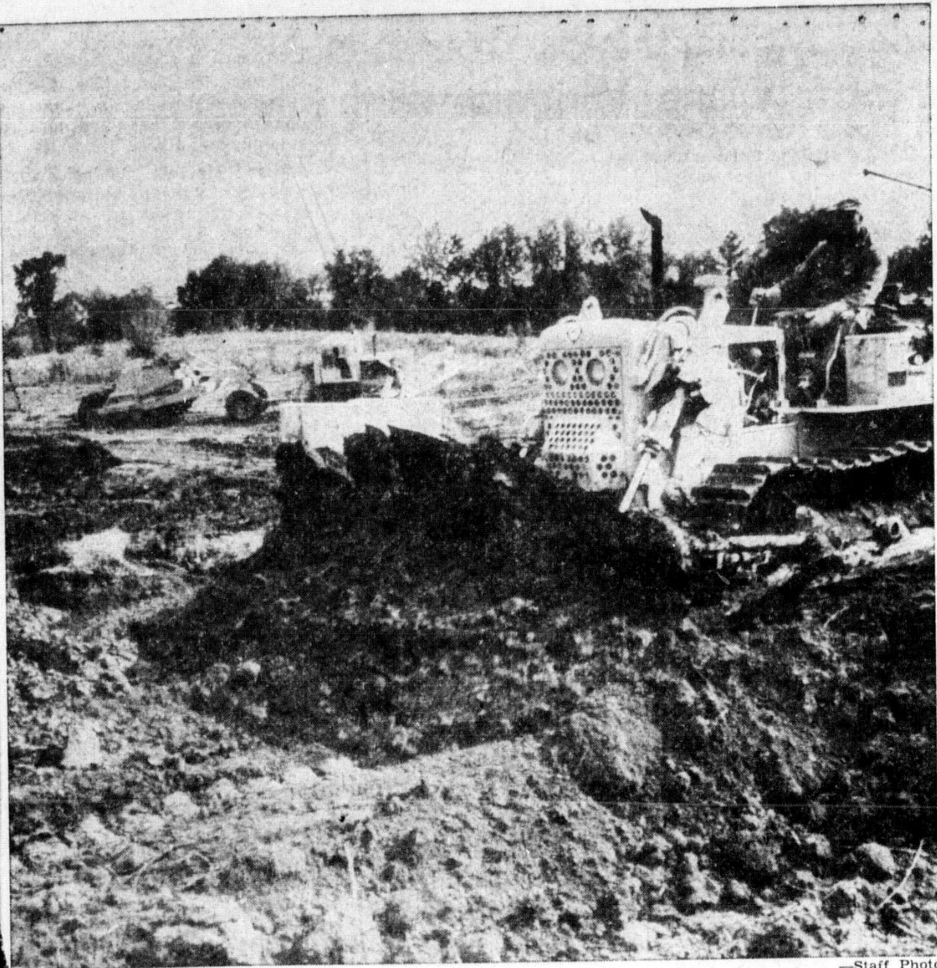
THE BURNS RESERVOIR , located on Lot 11, Concession 2 of the Township of Nassagaweya, is being constructed by the Halton Region Conservation Authority as a demonstration to show how a small dam can be built on farm property. Total cost of the project is about $4,000. Here large bulldozers are shown working on the project.
