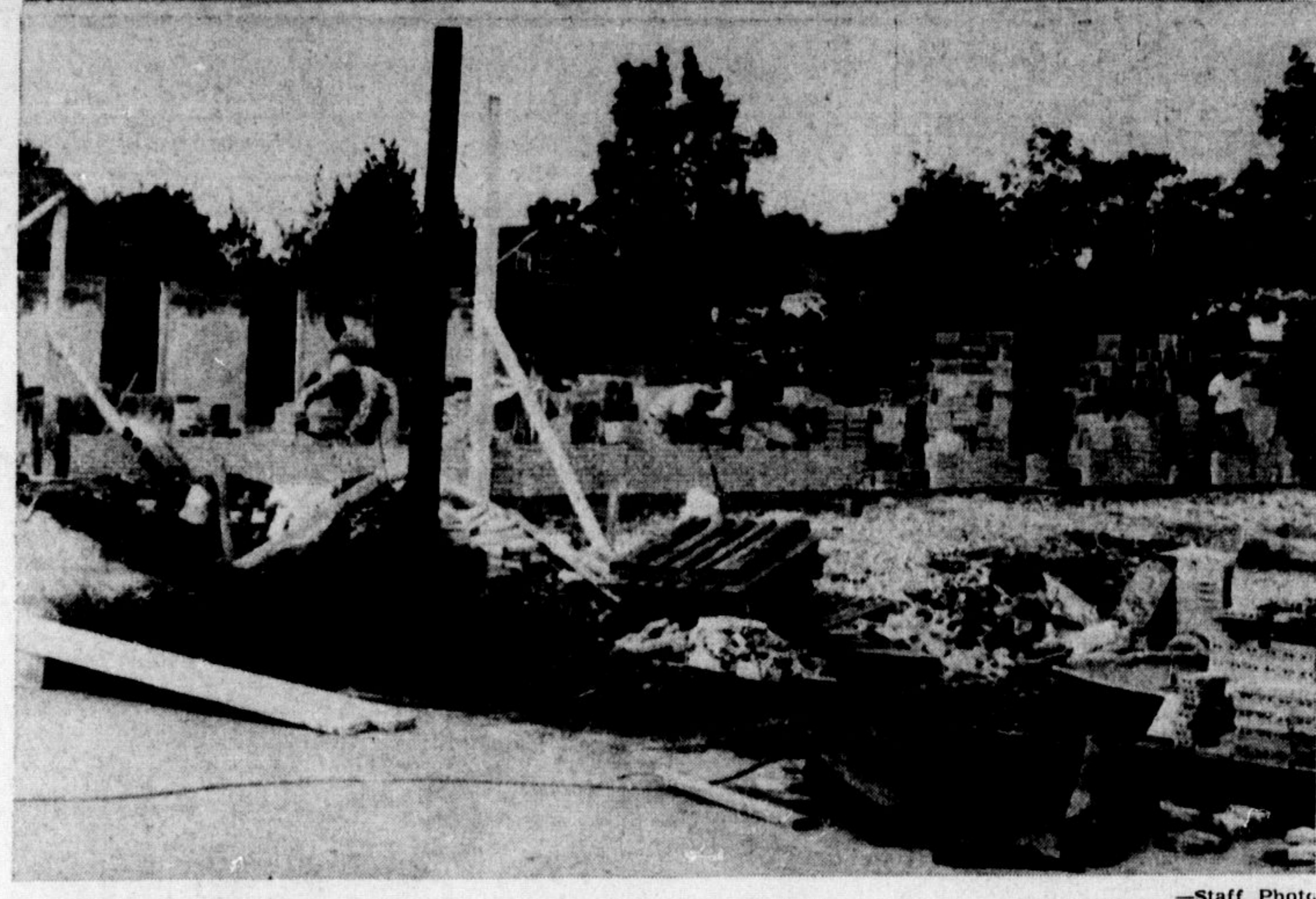
AN $80,000 ADDITION to the Holy Rosary Separate School is under construction and the board hopes to have it open for use in September. The four-room two-storey addition is the fourth addition to the school since it opened in 1954. One classroom will be a kindergarten, two are classrooms, and one is a general purpose room. It is being erected on the north side of the building, at the rear of the school.
