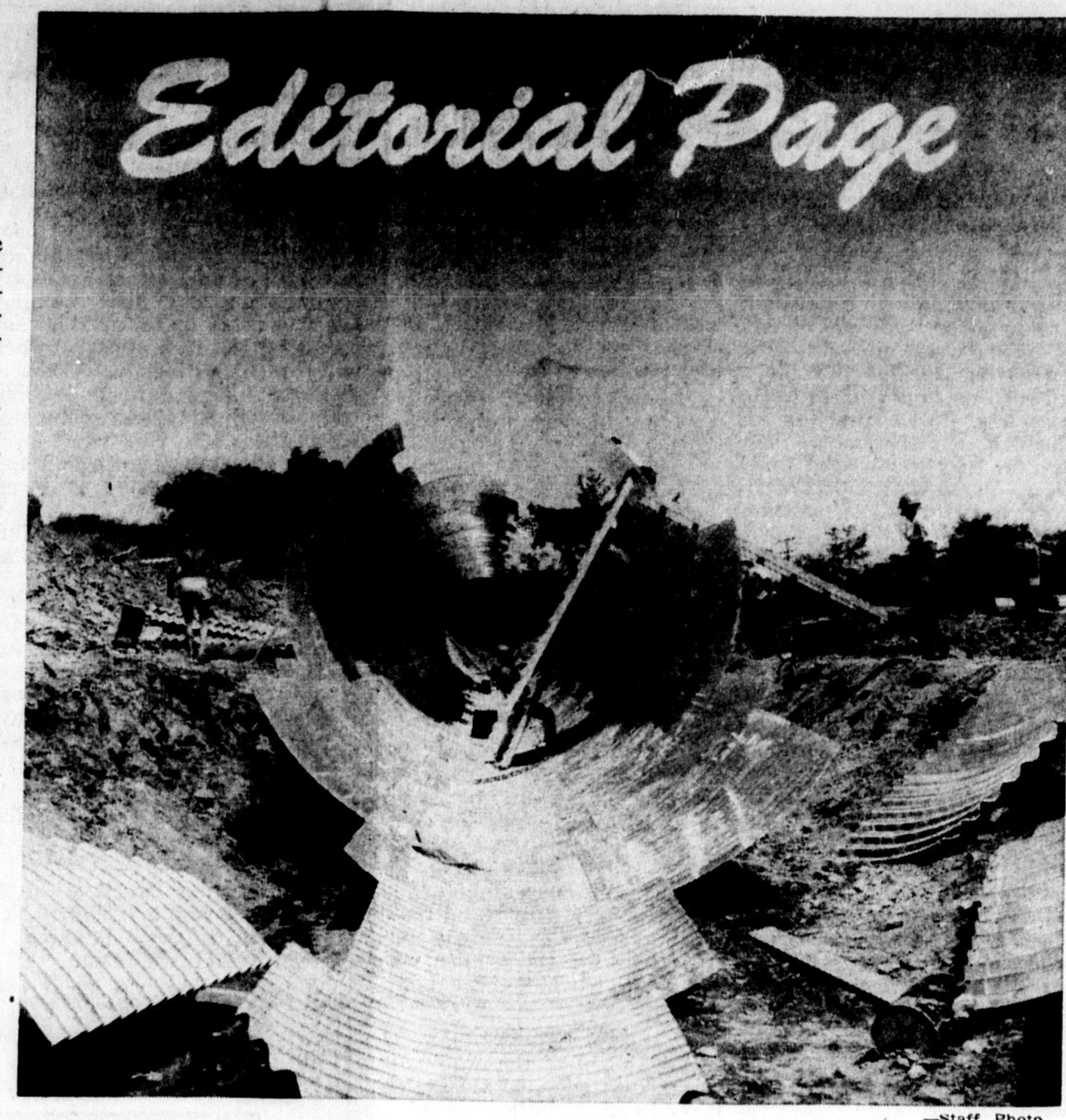
DWARFING MAN is this 14 foot culvert being installed in the C.N.R. by-pass wall that is surrounding the town. The culvert, 270 feet long, is located between the Base Line Road and Bronte St. It is one of two such culverts that will carry the stream through the railway embankment. The steel culvert with the necessary bolts will weigh 181 tons when completed.
