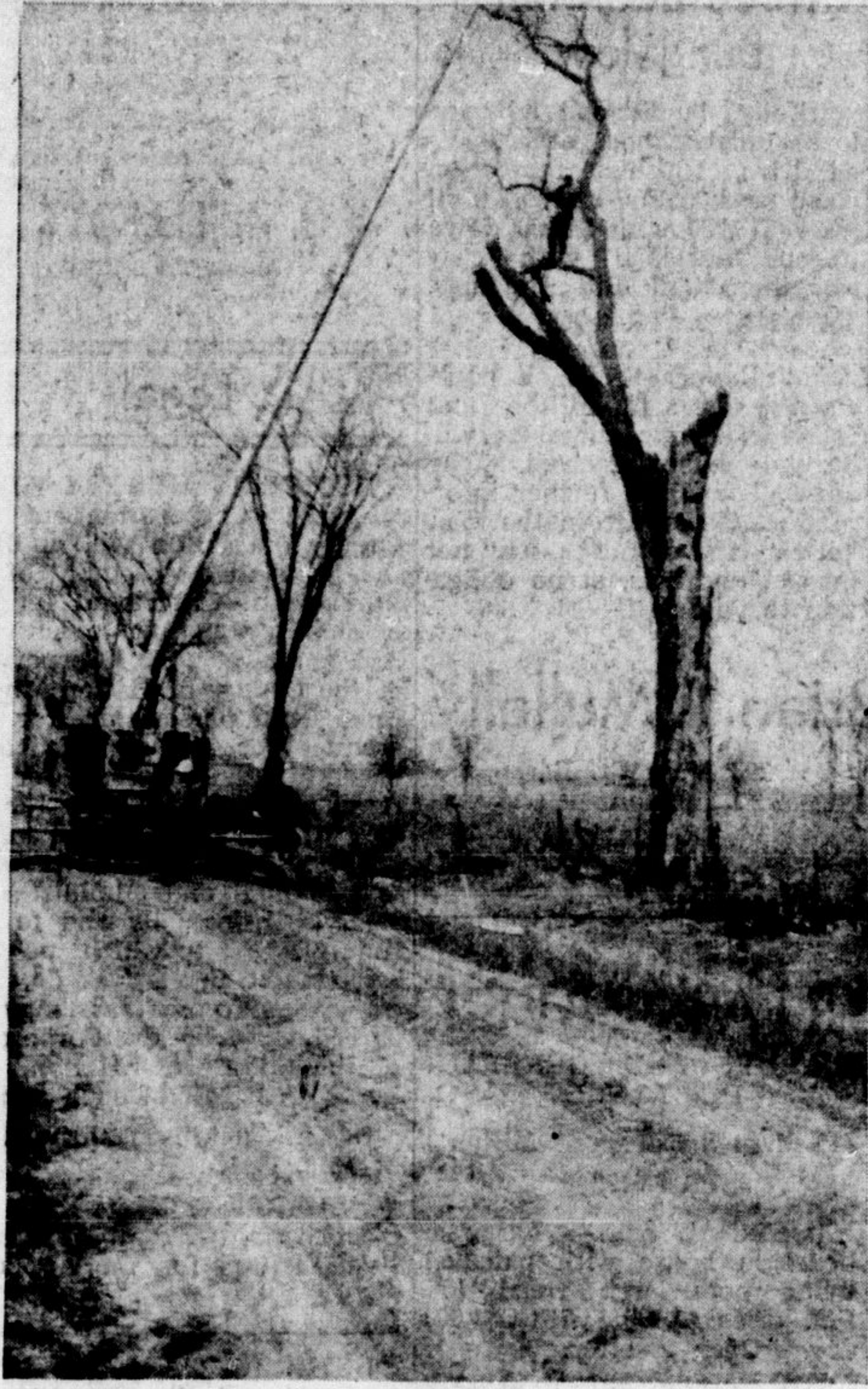
ONTARIO HYDRO ATLAS CRANE is shown on one of the roads in Vaughan Township being used to remove a diseased and hazardous elm tree. This tree was not safe for men to climb and the crane hoisted Hydro forestry workers into position so that they could cut limbs and main sections of the tree safely. The only live branches of this tree extended directly over rural power lines and this presented a possible hazard to service for rural customers.
