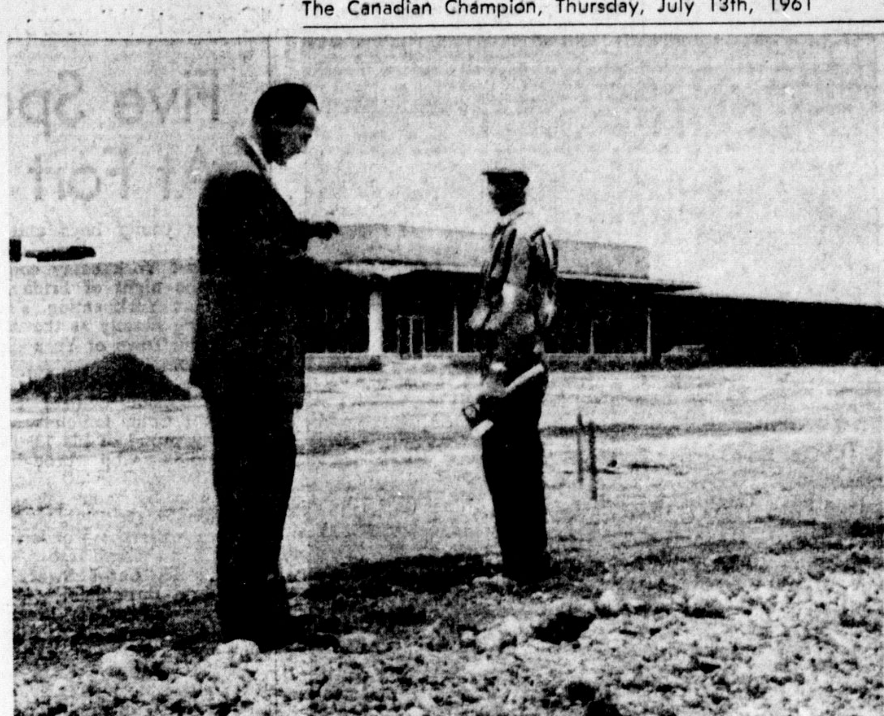
THE FIRST PHASE of the Milton Plaza is well on its way to completion. This $300,000 section includes a Loblaw's store and 10 smaller stores with a total of 20,000 square feet. John Tamai of Oakview Developments who hopes to have the shopping centre open shortly, gives instructions to Gino Gaeton concerning the 500 car capacity parking lot.
