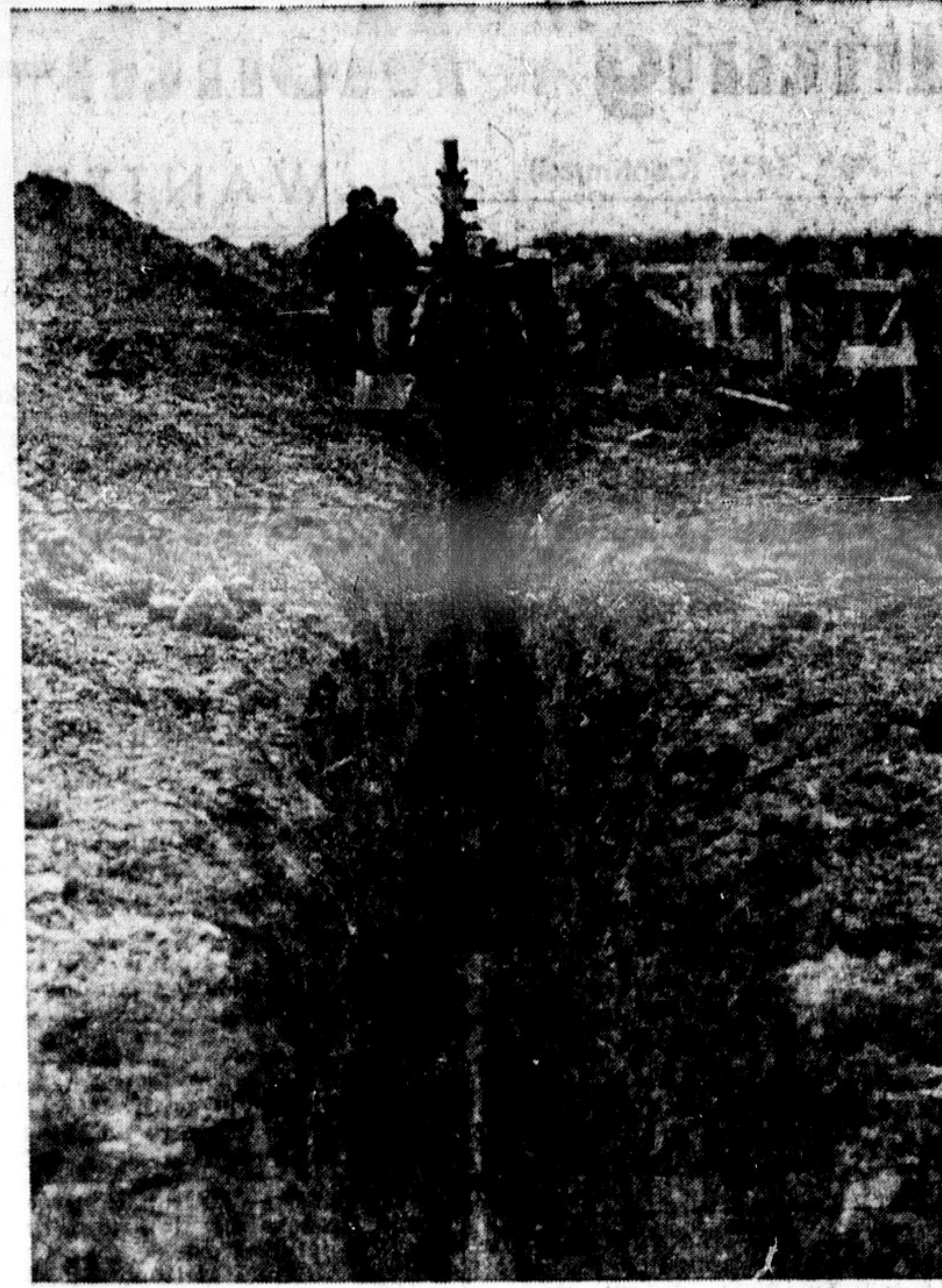
WATER LINE into the site of the Milton District Hospital is nearly completed, and water service should soon be turned on. Next comes the installation of the sewers. Above, workmen are shown laying the lengths of pipes into the hole as the trenching machine prepares the trench.
