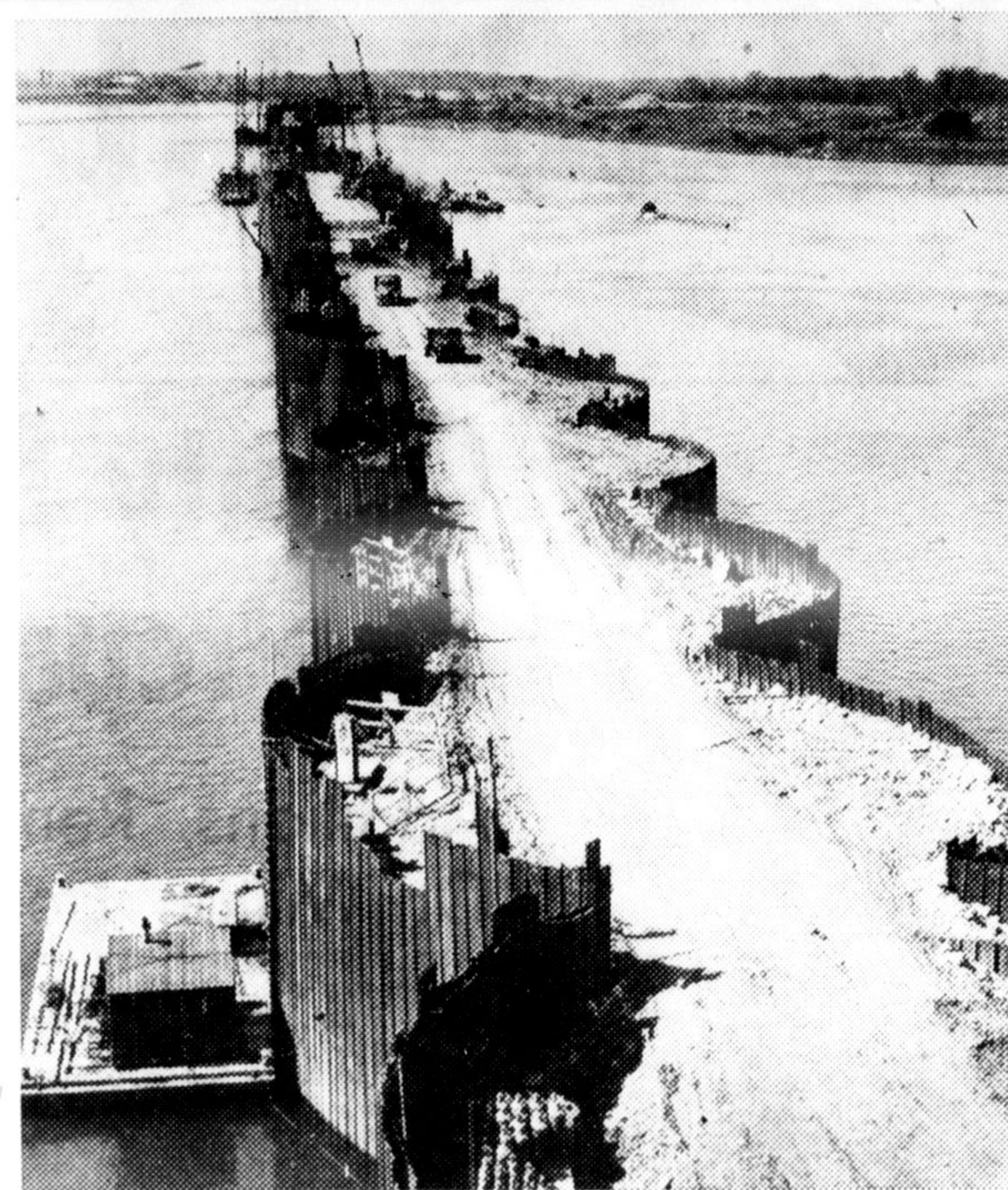
POWER IN THE MAKING —Men and machines at work during construction of a 4,500-foot long cofferdam which now spans the north channel of the St. Lawrence River from a point on the Canadian mainland near Cornwall to Barnhart Island, on the United States side. With the completion in June of the structure shown above, together with a second cofferdam some two miles upstream between Sheek and Barnhart Islands, dewatering of the enclosed area was able to proceed. Some 650,000,000 gallons of water has been pumped out to permit construction of the Canadian powerhouse to proceed "in the dry."
