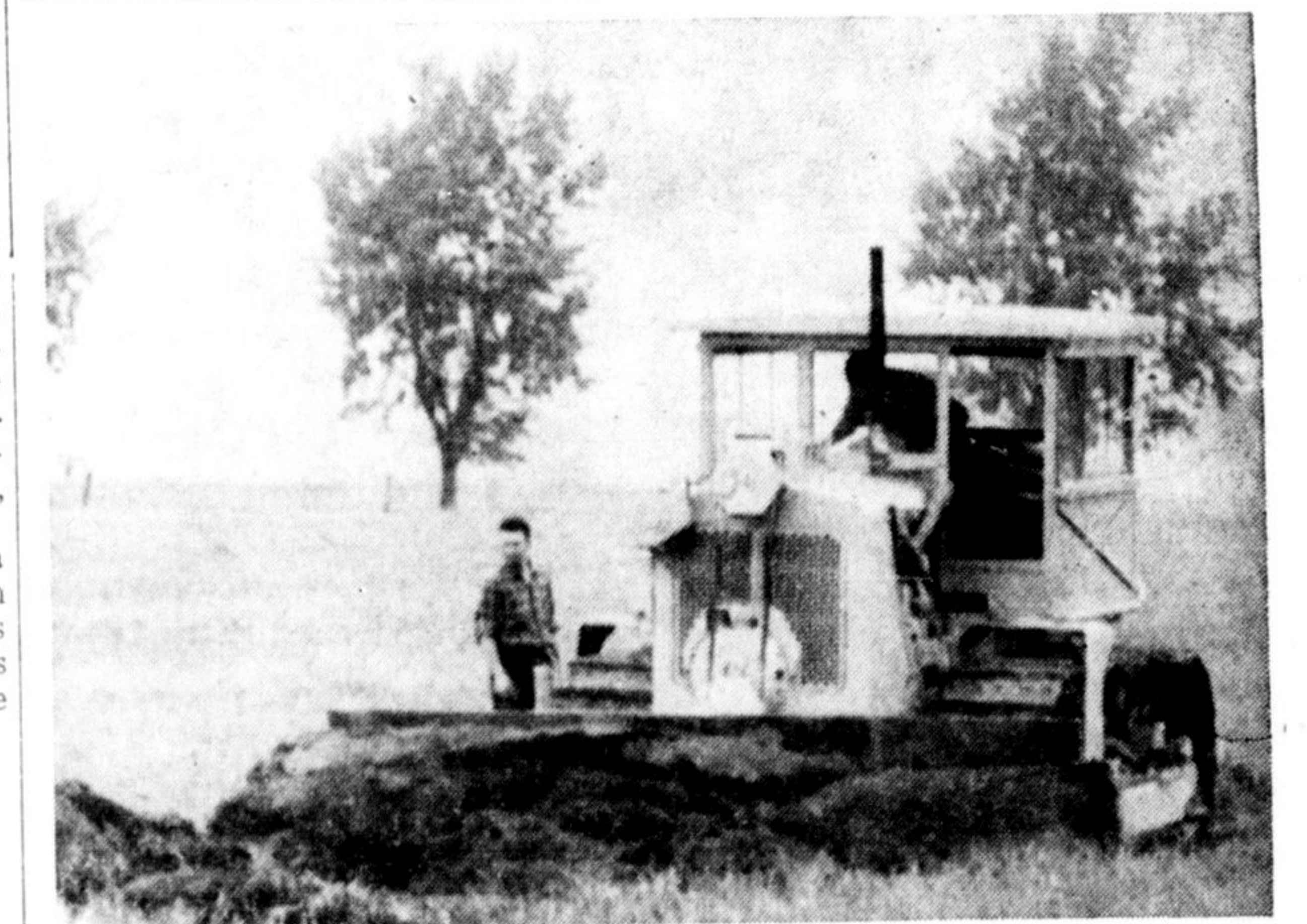
RIPPING INTO THE SOIL to remove the first sods at the site of the Canadian Meter Co. yesterday (Wednesday) is this bulldozer of the Frid Construction Co. who have the contract for construction of the 35,000 square foot plant. The Meter Co. is presently located in Hamilton and will be transferring their operations to Milton.
