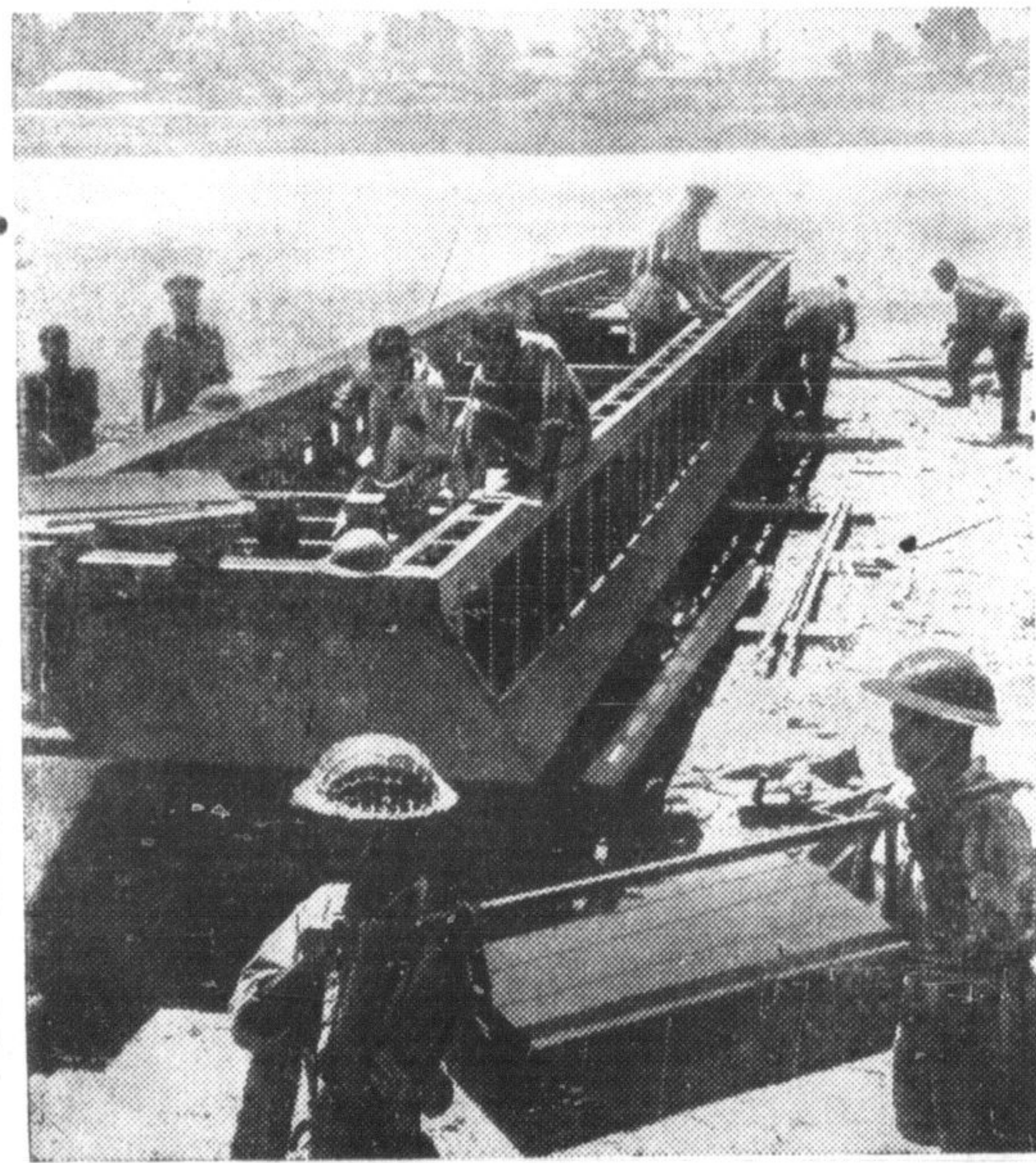
A new type of pontoon bridge is now under construction in Arakan. All its components are prefabricated and can be transported by jeep and assembled in a very short time.
