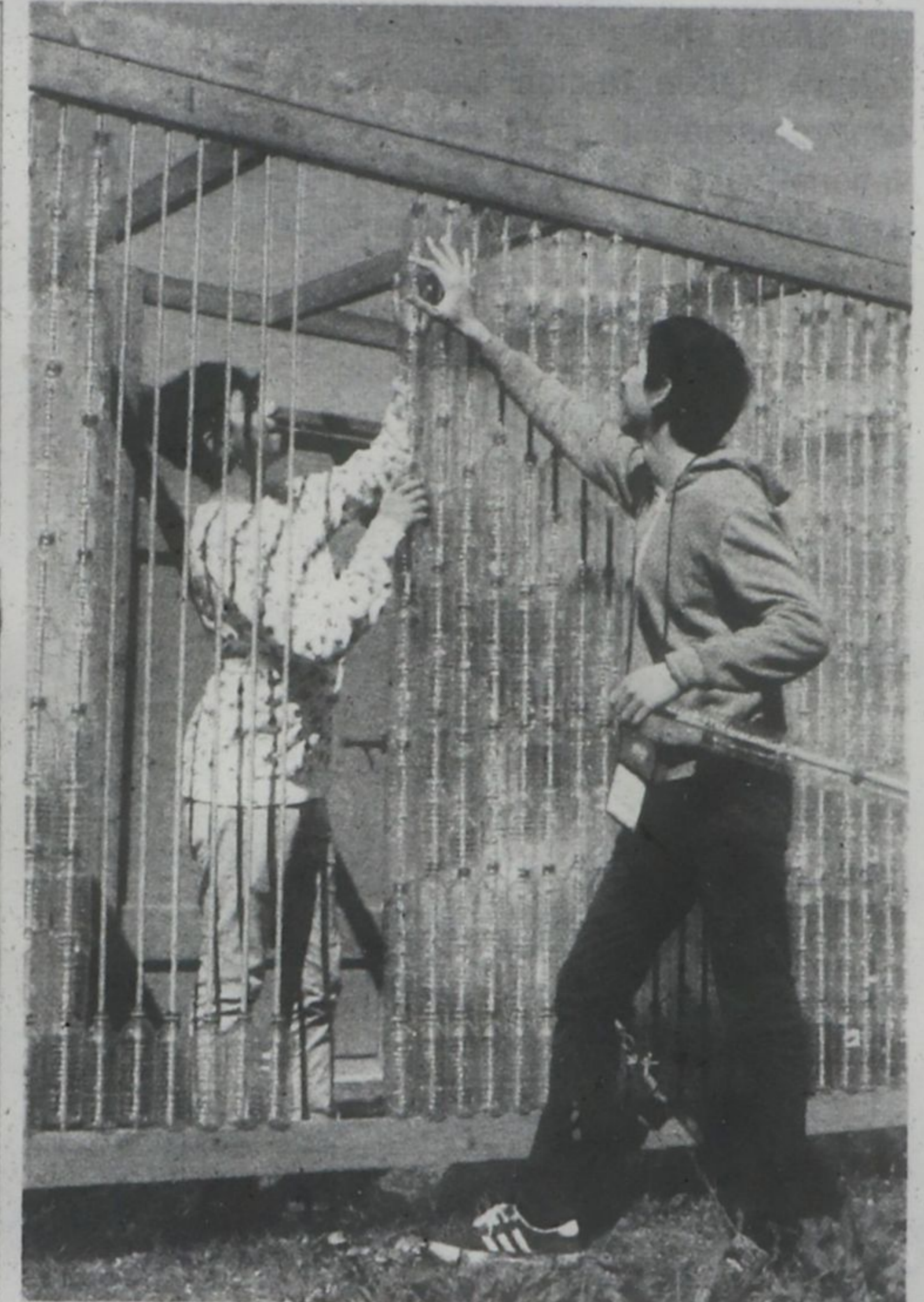
Volunteers and staff of Country Heritage Park teamed-up to build a greenhouse out of discarded plastic bottles. The environmentally-friendly initiative was also part of Milton Culture Days. Volunteers Suhaib Aldada, 15, (left) installs another one of the steel rods/ plastic water bottle pieces, with help from Amro Alattar, 16, that form the greenhouse walls.
