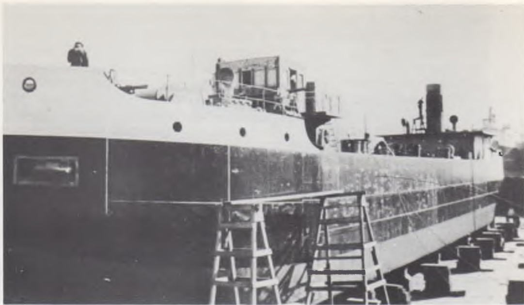
BRUCE HUDSON is converted to a steamer in the Muir Bros. drydock at Port Dalhousie, winter 1938-1939. Photo courtesy Lorne Joyce.
