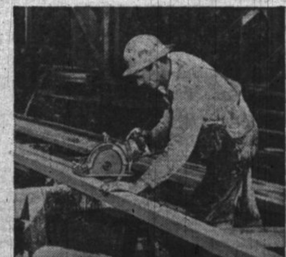
Portable Electric skill saws help to cut days from production schedules of minesweepers which are constructed almost entirely of wood.
