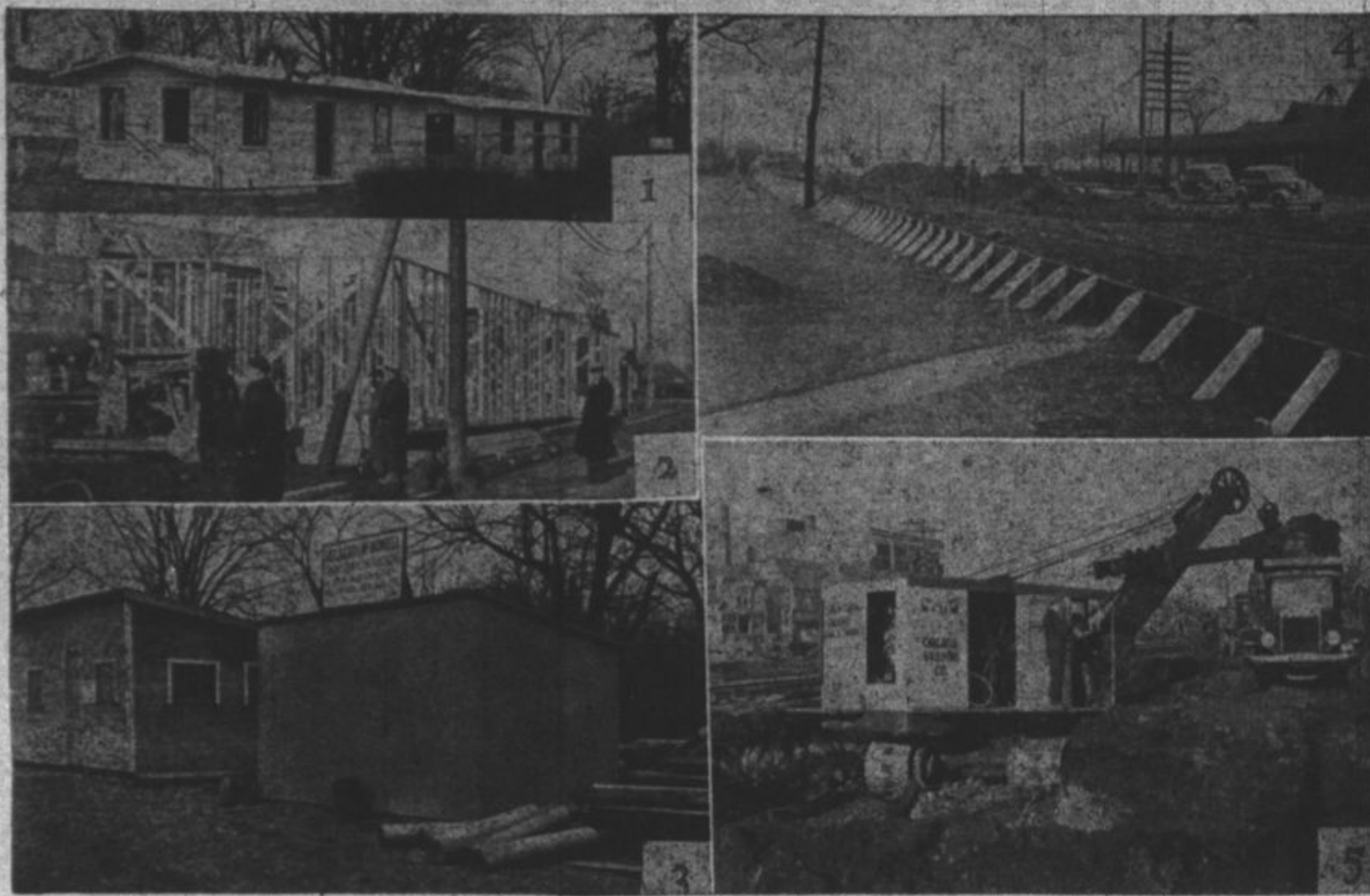
Work was started last week on the grade separation from South avenue, Glencoe, through Winnetka to the southern limits of the project a short distance north of Kenilworth avenue. The foregoing pictures are:
