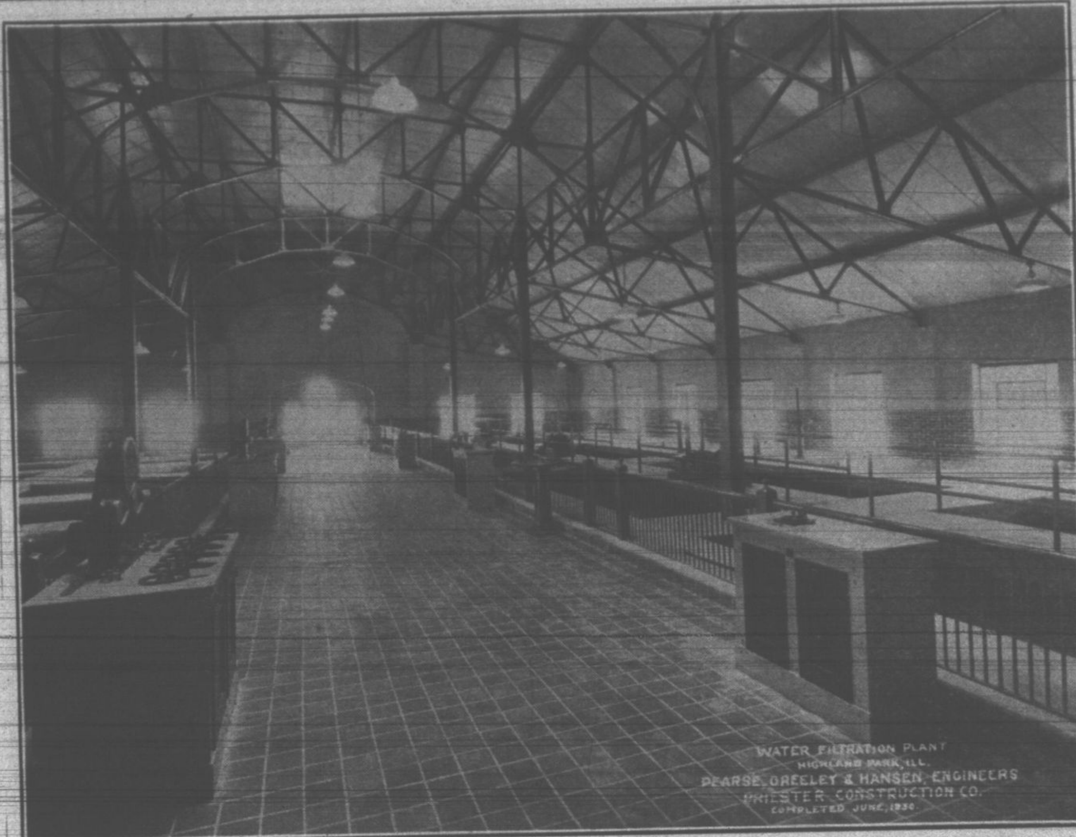
The Operating Floor of the Filter Room showing the Control Tables. The Mixing Basins are on the right.
